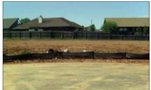
Photo courtesy of the City of Oklahoma City Stormwater Program
