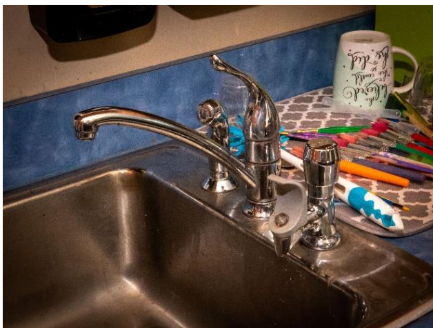
The image above is of a Classroom Faucet (CF) and Drinking Water Fountain (DW) that were sampled at a school. There were multiple schools with two (2) fixtures on each sink. These are often found in schools built prior to 1980.
