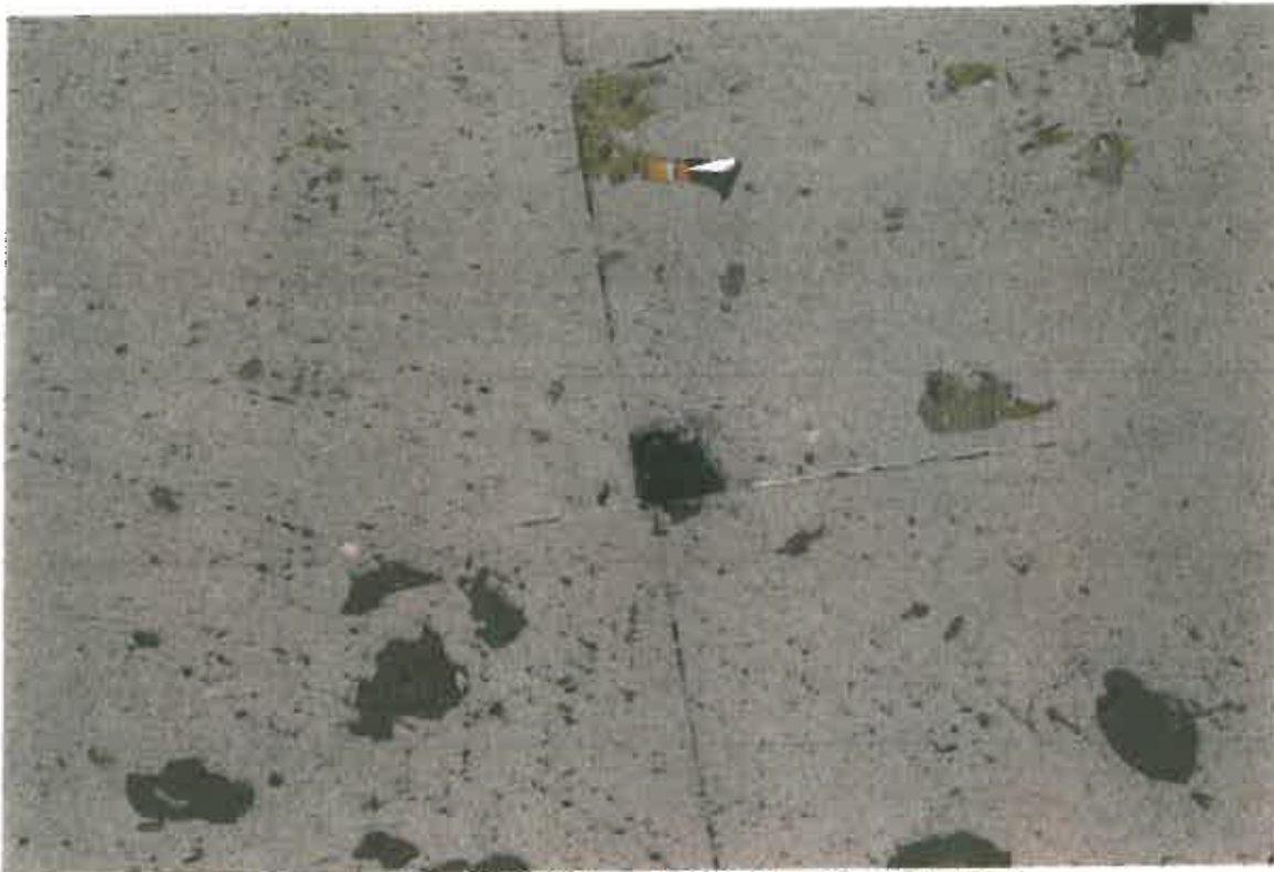
Samples 05A, 05B, 06A and 06B (Contain Asbestos)
