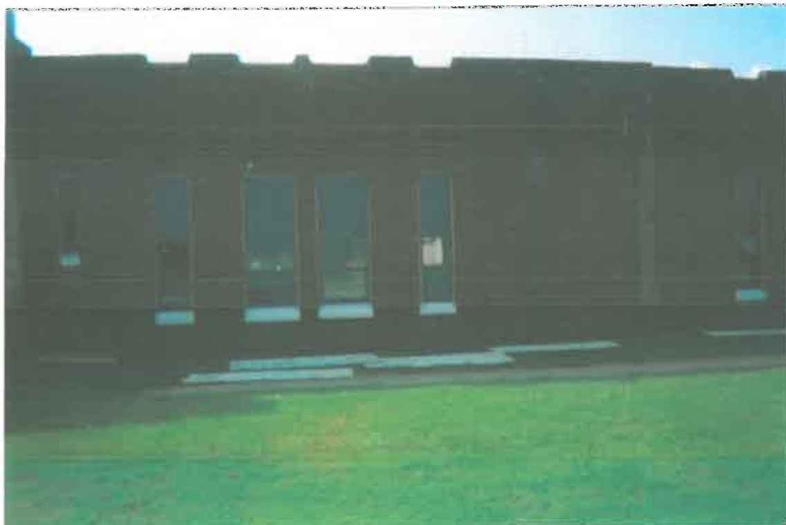
Armory exterior - New doors and windows - window sills and door frame abated.
