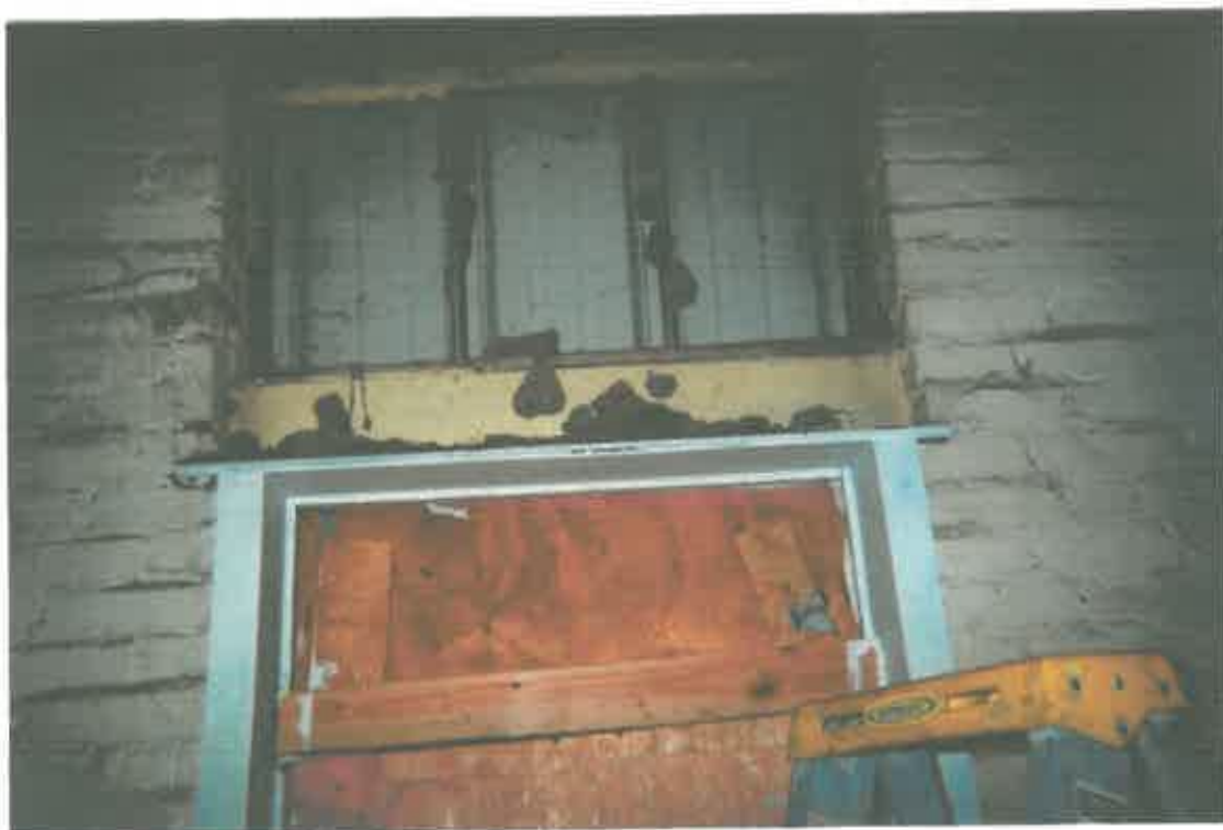
Window sill in armory prior to abatement.
