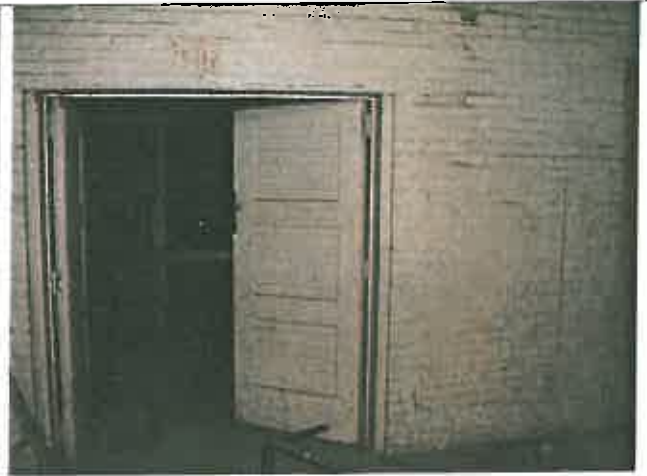
Reading 16, Room 1, Side A, Wood door & casing
