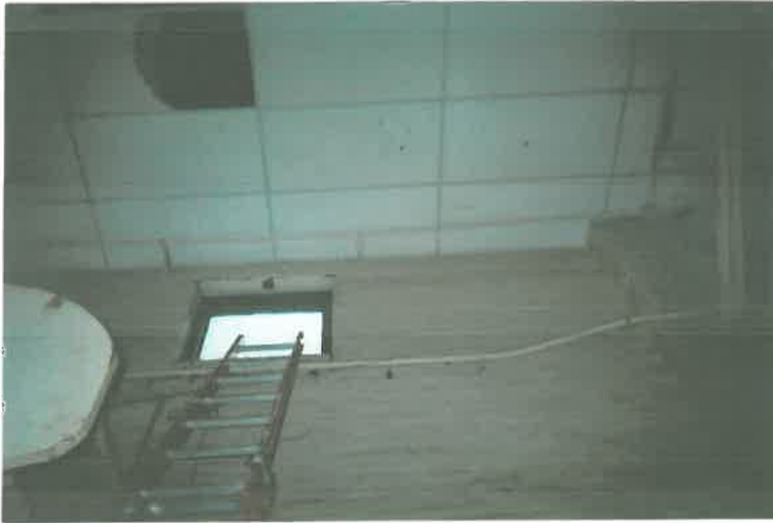
Window sill in armory prior to abatement.
