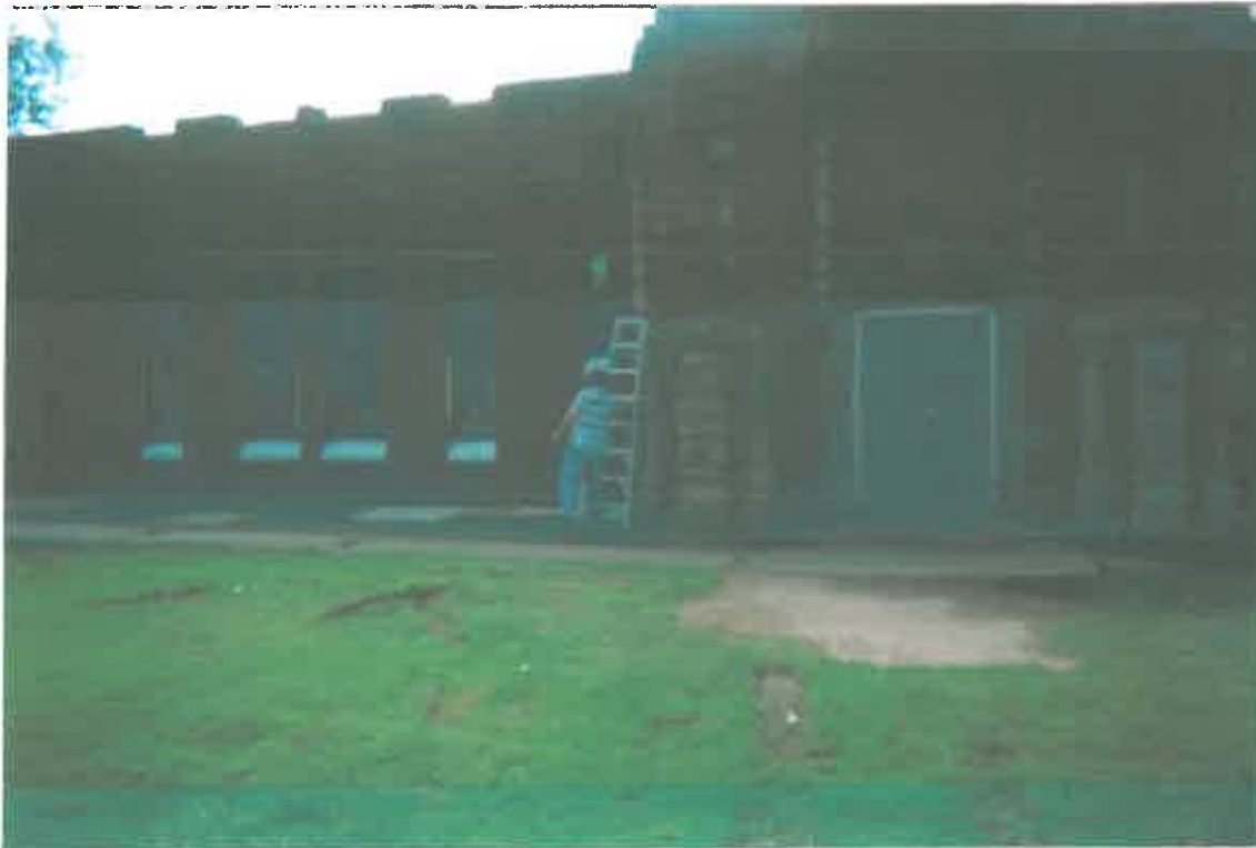
Armory exterior - New doors and windows - window sills and door frame abated.
