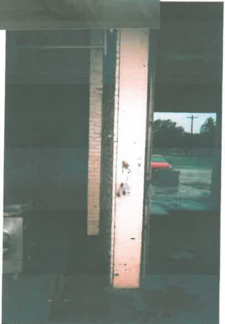
Another door frame before abatement.
