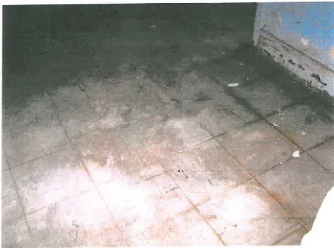
Samples 08A, 08B, 09A and 09B (Contain Asbestos)
