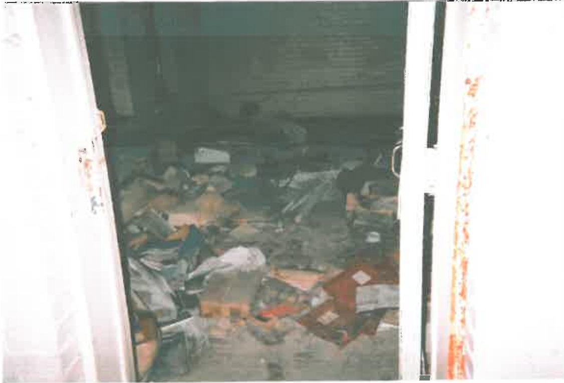
Non-ACM waste in armory room.
