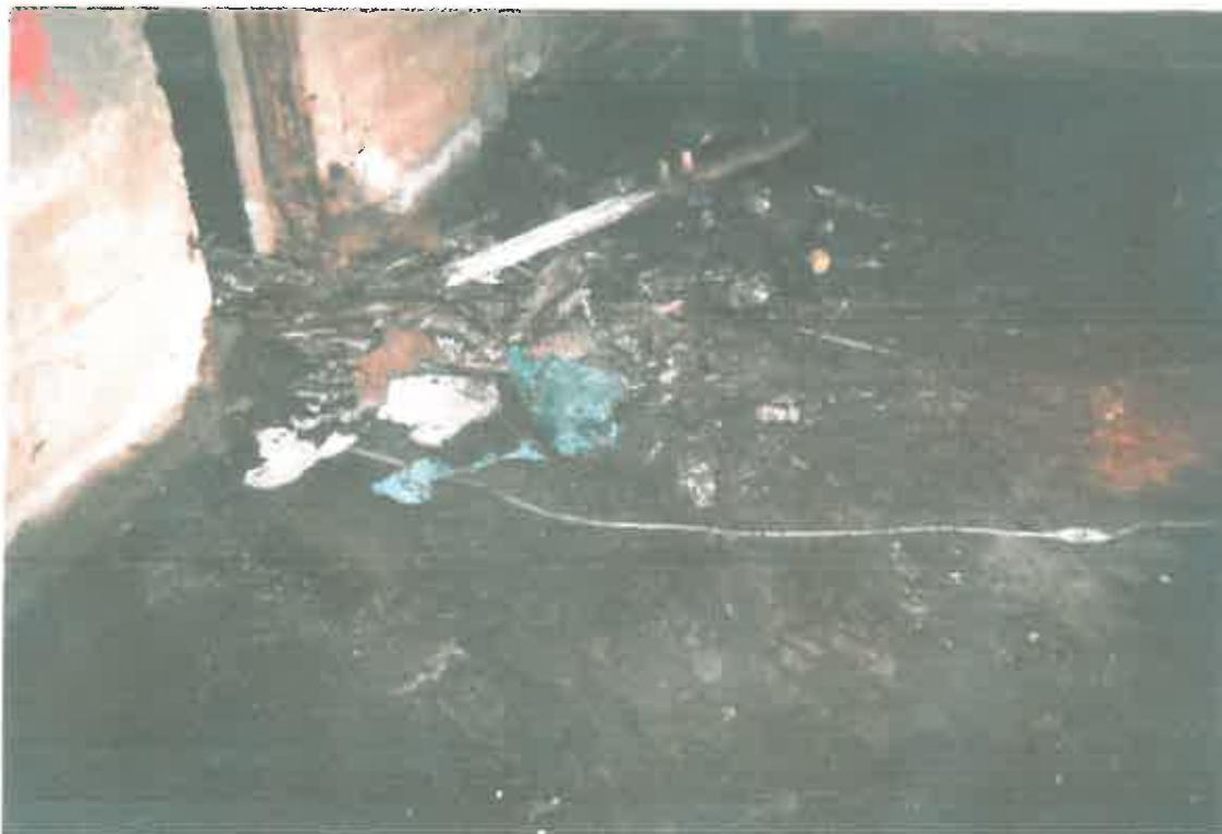
Non-ACM waste in armory room.
