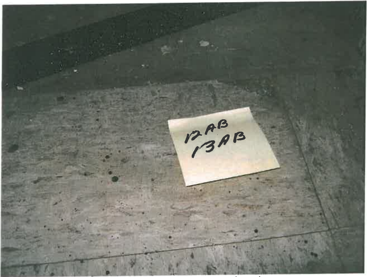
Samples 12A and 12B (Contain Asbestos)
