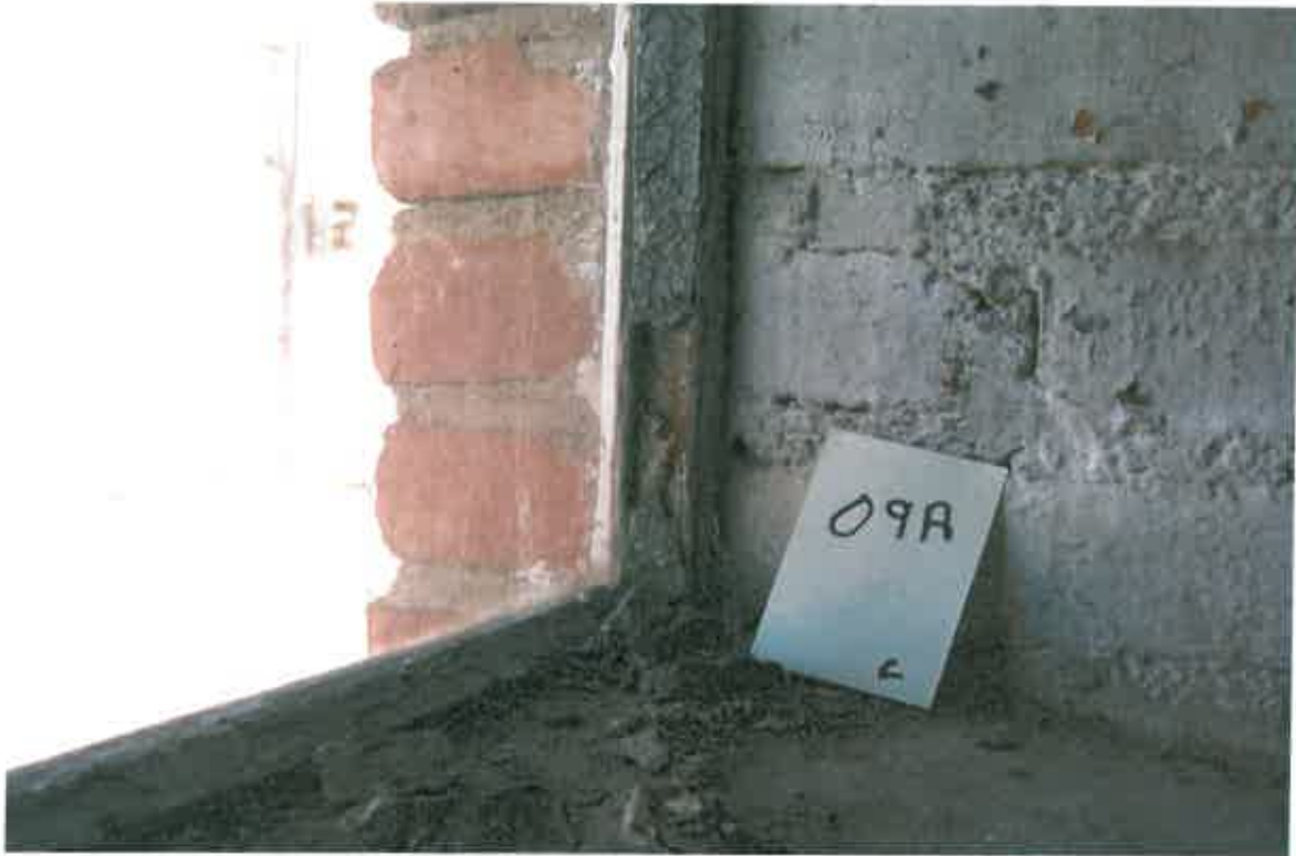
Friable Asbestos Containing Window Caulking (Sample # WA-09A)
