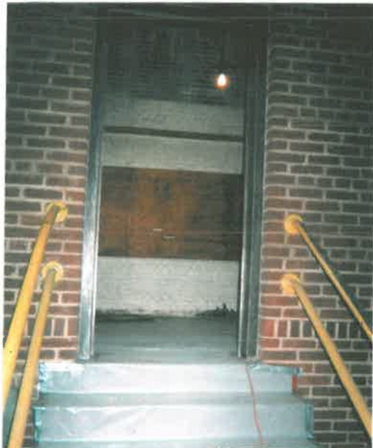
HAND RAILS AND STEPS - BEFORE ABATEMENT
