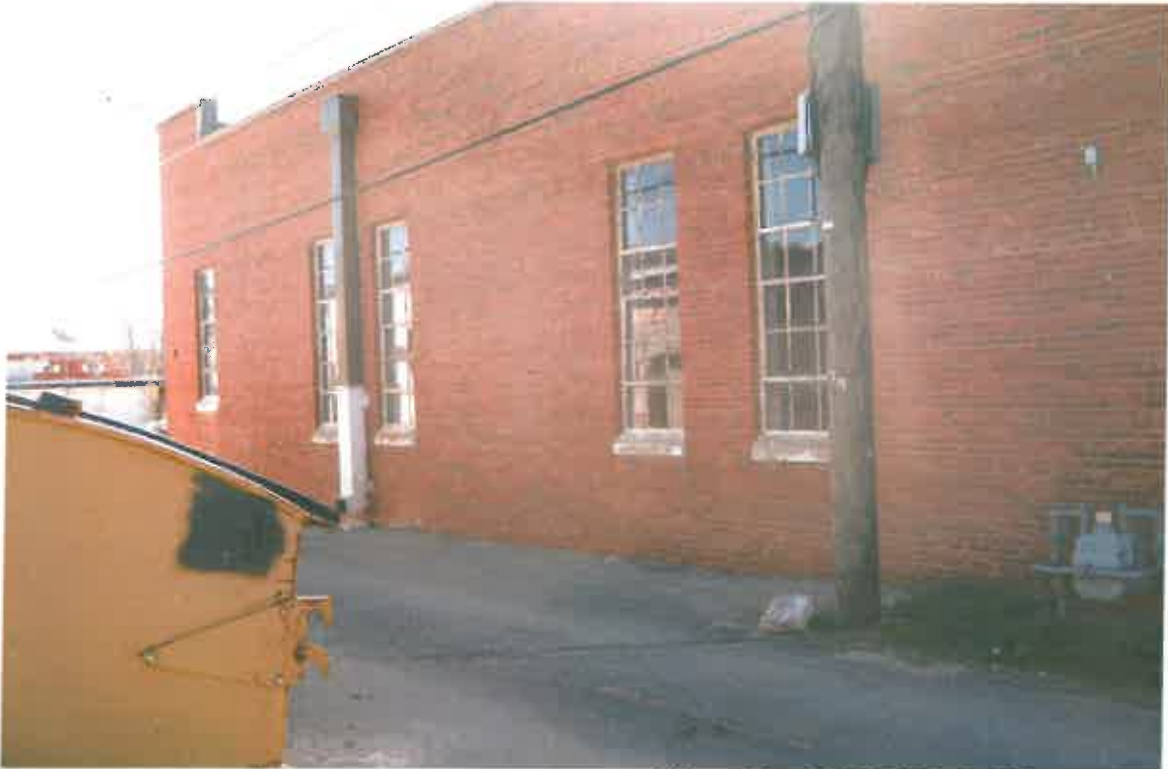
Friable Asbestos Containing Window Caulking, East Half of North Side
