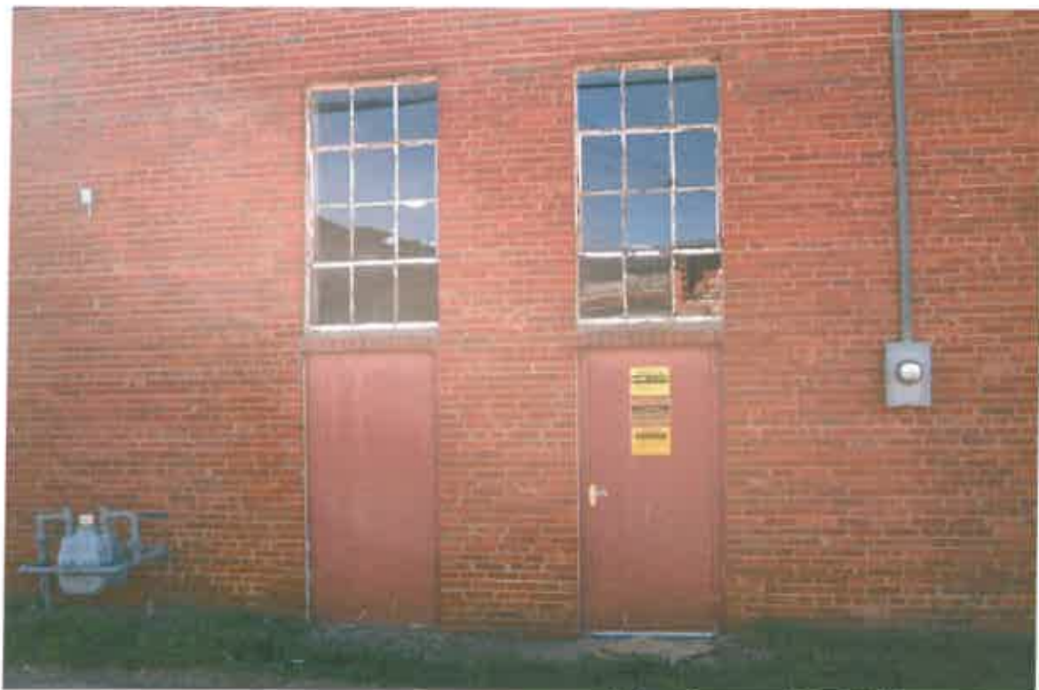
Friable Asbestos Containing Window Caulking, Center of North Side
