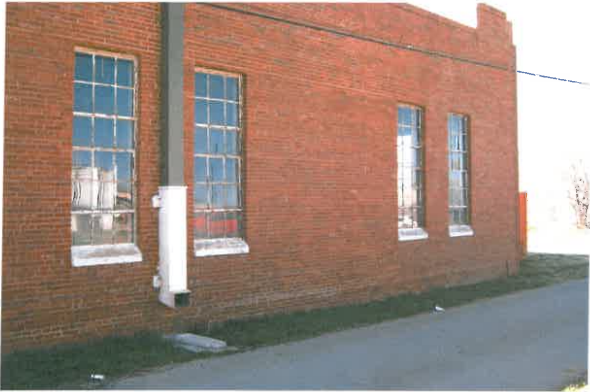
Friable Asbestos Containing Window Caulking, West Half of North Side
