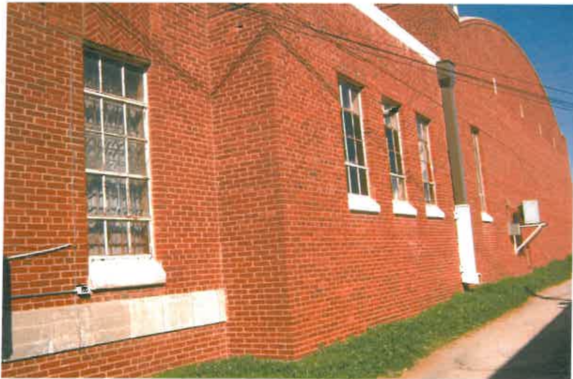
Friable Asbestos Containing Window Caulking, East Side
