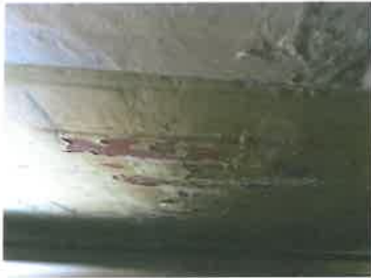
Photo #1: Yellow Paint Behind Range
