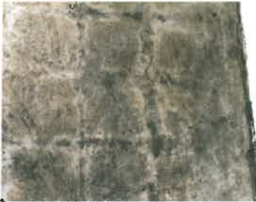
Photo #1: Mastic Removal Remnants
