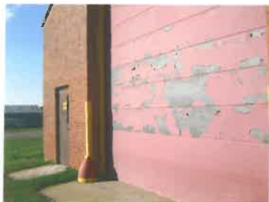
Photo #10: Red-painted rollup doors - LBP.
