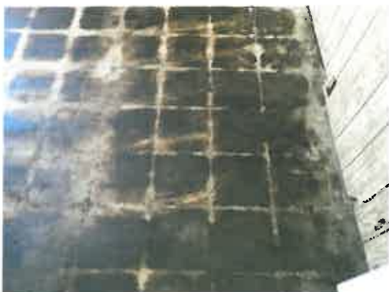
Photo #5: Mastic Removal Remnants
