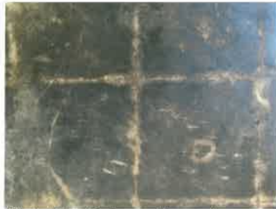
Photo #4: Mastic Removal Remnants
