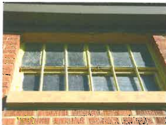
Photo #16: Yellow-painted wood window lintels on Sides B & C - LBP.
