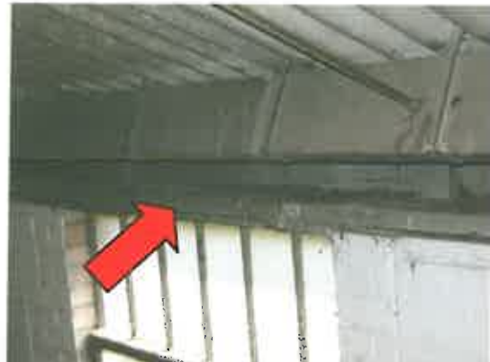
Photo #8: Wood boards at the top of the wall, Room 16 - LBP.
