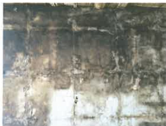
Photo #6: Mastic Removal Remnants
