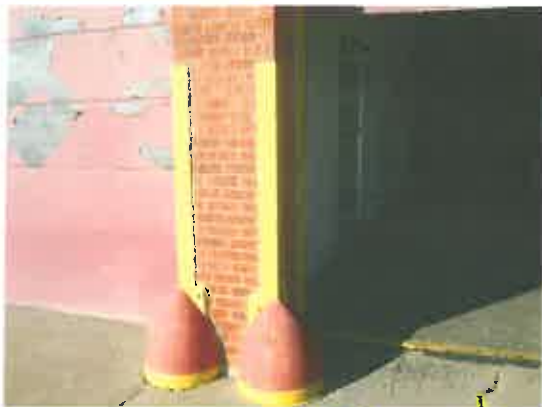
Photo #15: Yellow-painted metal edge protectors, Sides A & D - LBP.
