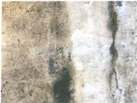
Photo #3: Mastic Removal Remnants
