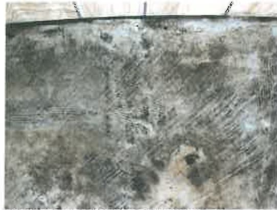
Photo #2: Mastic Removal Remnants
