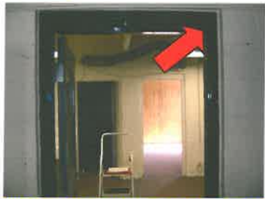
Photo #4: Black painted metal door frame, Room in 15 - LBP.
