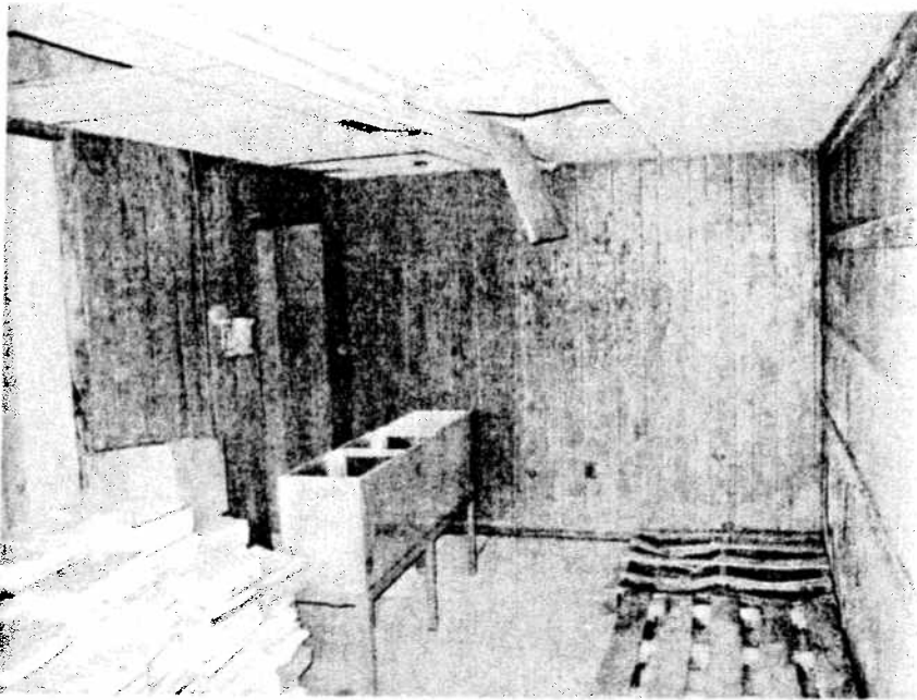
Figure 9: Room off northeast side of the drill floor showing water damage.
