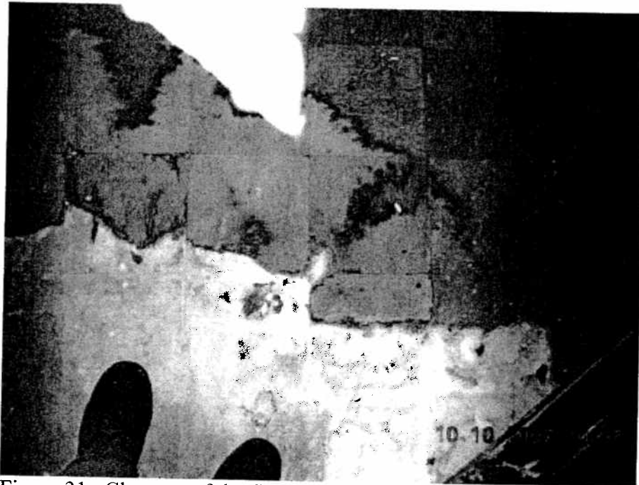
Figure 31. Close-up of the floor tiles seen in figure 29. The 9 inch tiles are chipping and crumbling and likely contain asbestos.
