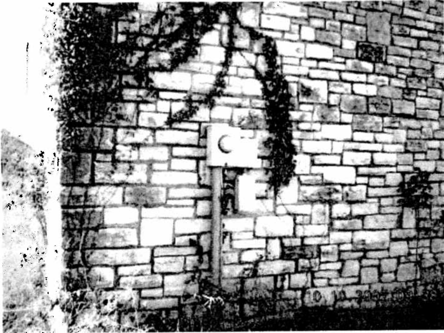
Figure 5. Electric meter box on northeast corner of armory.
