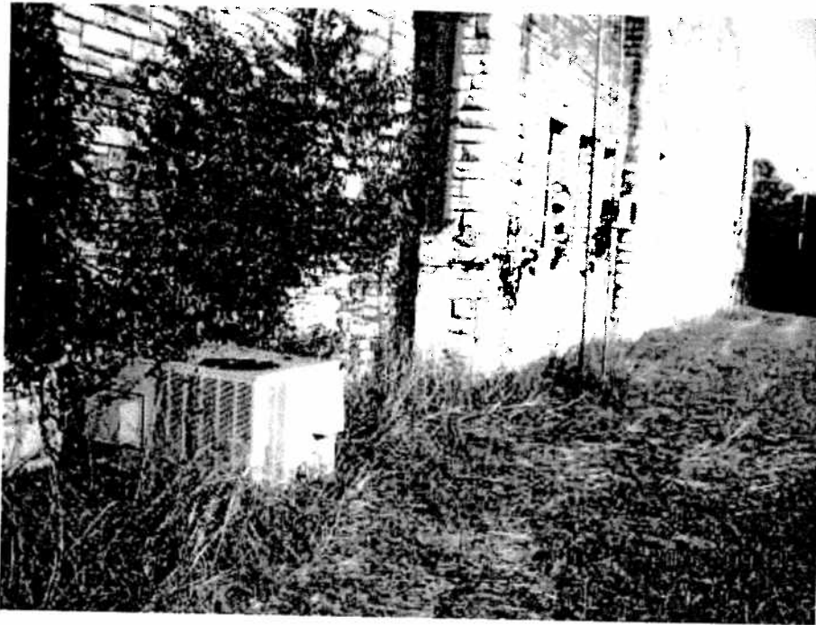
Figure 7. Central air-conditioner for offices in south part of the armory. Located near the southeast corner of the armory.
