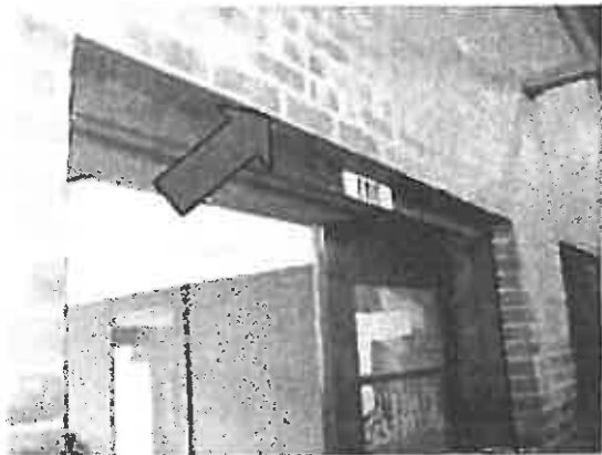
Photo #12: Brown painted metal door lintel associated with Room 2 - LBP.
