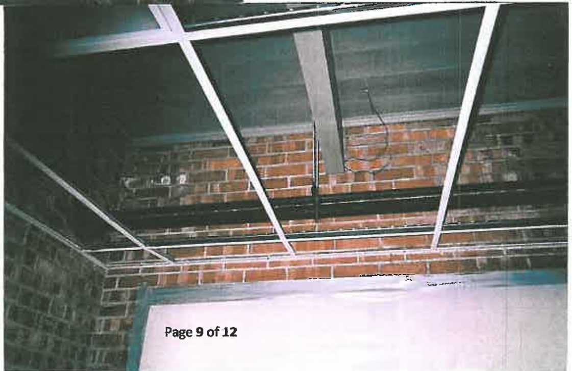
Piping post abatement
