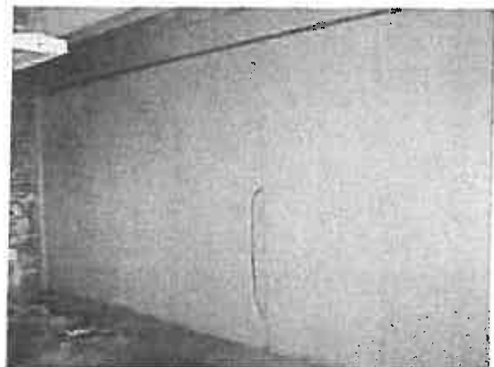
Photo #16: Gray painted wood wall in Room 7 - LBP.
