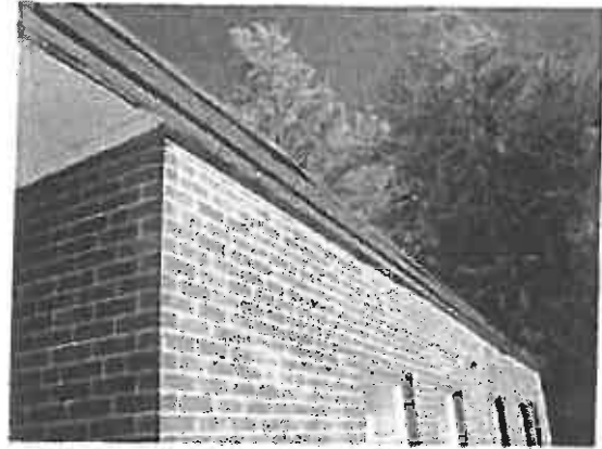
Photo #2: View of black painted fascia on the exterior of the armory building - LBP.
