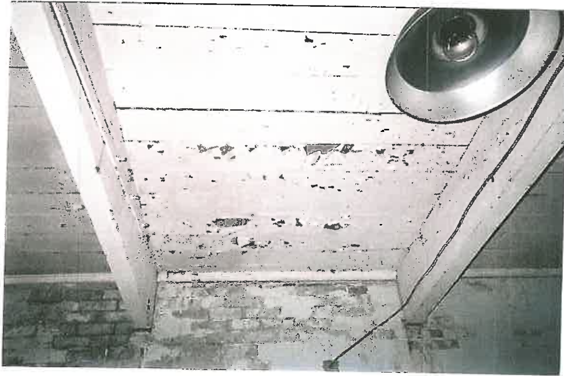
Ceiling - loose/peeling paint prior to abatement
