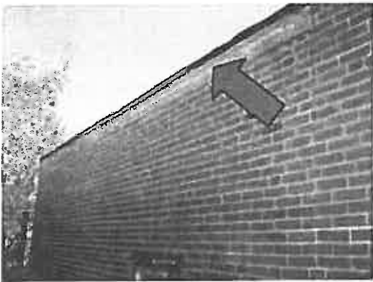
Photo #9: View of white painted wood fascia board - LBP.
