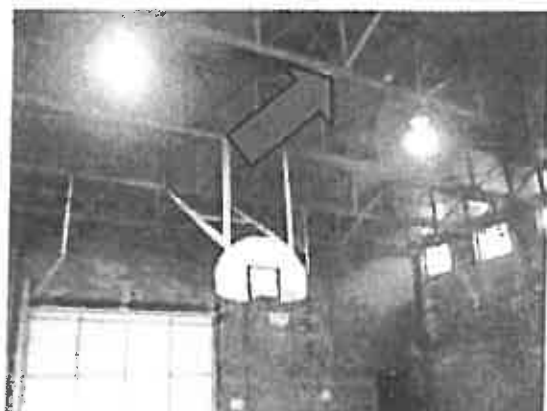
Photo #18: Gray painted trusses in Room 1 - LBP.
