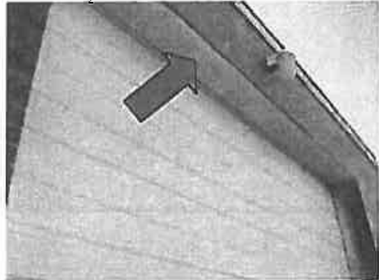
Photo #8: White painted roll-up door lintel on the exterior of the armory building - LBP.
