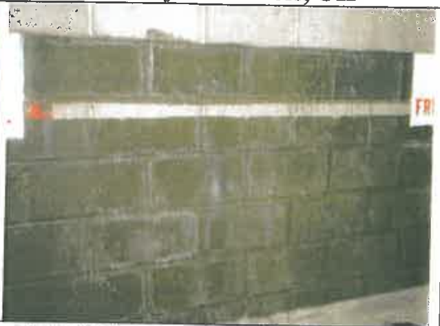
Photo #8: A gray portion of interior concrete wall on the north side of Building 2 –LBP.
