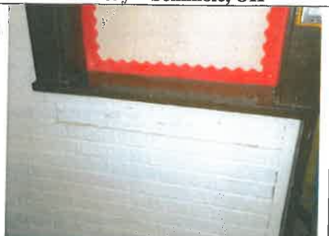
Photo #2: Brown pass-through window – LBP.
