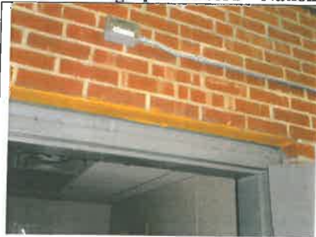
Photo #7: Yellow lintel in Room 19 –LBP
