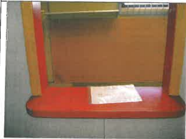
Photo #9: Yellow window frame trim in Room 2 –LBP
