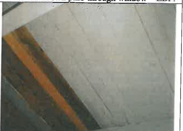
Photo #4: Gray ceiling deck – LBP.
