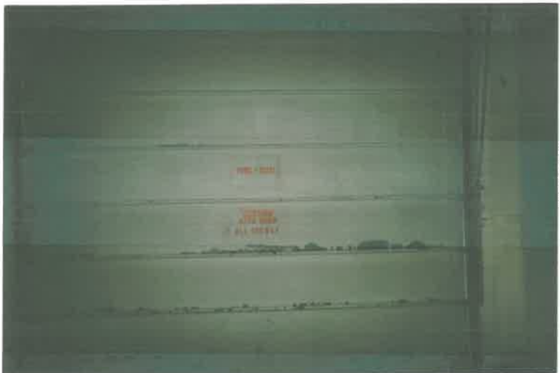
LOOSE AND PEELING PAINT - OVERHEAD DOOR
