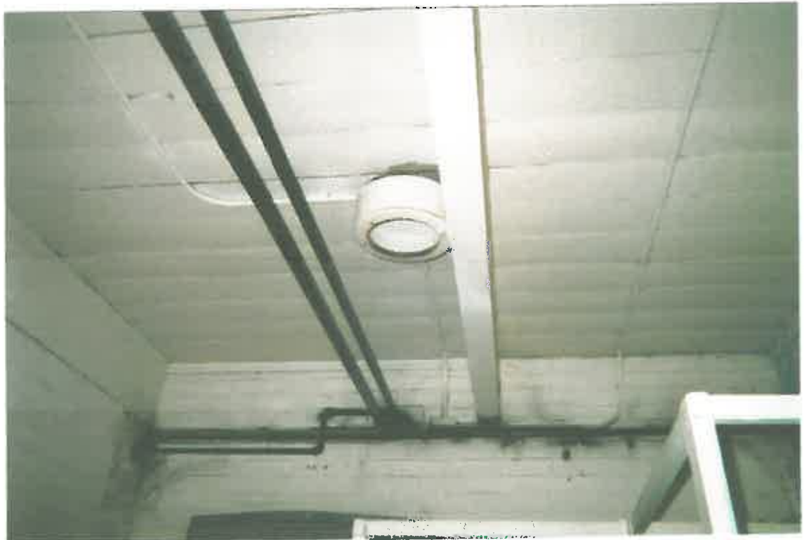
ABATED PIPE INSULATION
