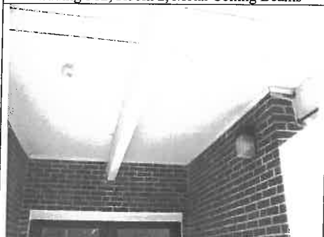
Reading 785, Exterior, Wood Porch Beams Reading 786, Exterior, Wood Porch Ceiling
