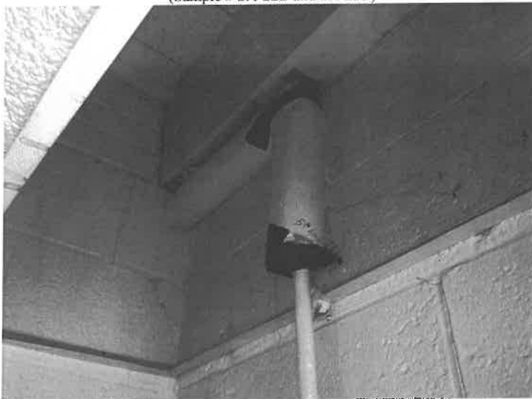
Friable Asbestos Containing Thermal Pipe & Fitting Insulation (Sample # SA-22C and SA-23C)
