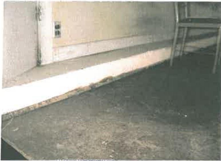
Figure 3. White Concrete Ledge - Room 27 (Side C)
