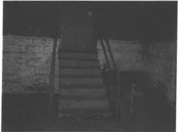
Photo: 14) Post Lead-Based Paint Abatement of Stair Rail, New Door and Door Frame.
