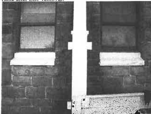
Photo: 11) Post Lead Abatement; Downspout and Window Sill Sealed with Approved Encapsulant.
