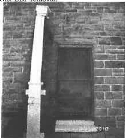
Photo: 11) Post Lead Abatement; Downspout and Window Sill Sealed with Approved Encapsulant.
