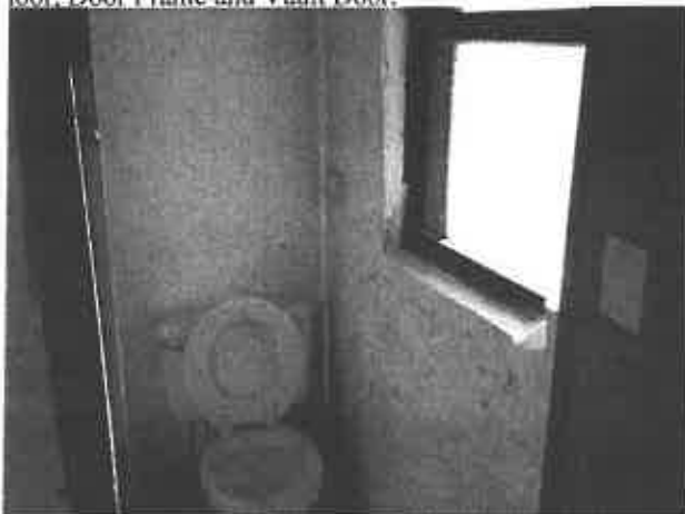
Photo: 17) Post Lead Abatement; Primed Door Frame after LBP Removal and Encapsulated Walls.
