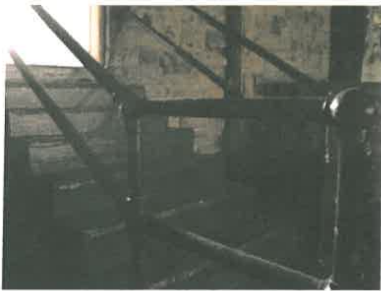
Figure 2. Browa Stair Rail- Room 27 (Side C - South)
