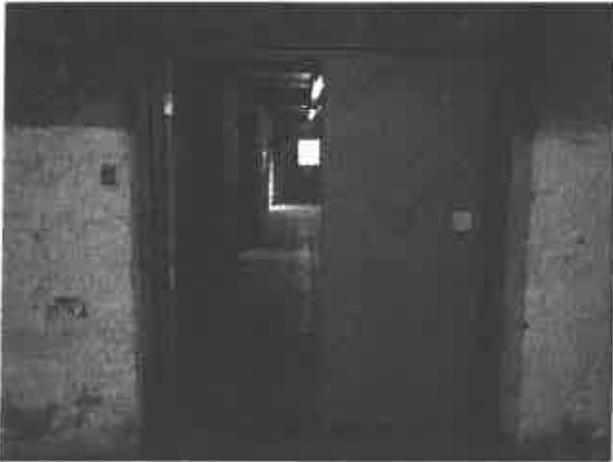
Photo: 13) Post Lead-Based Paint Abatement. New Door and Primed Door Frame after LBP Removal.
