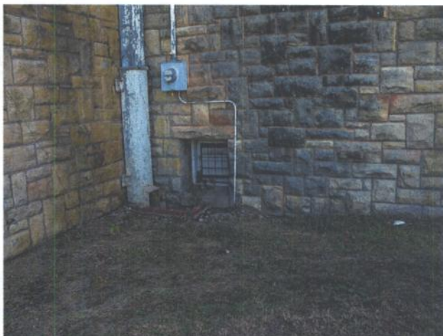
Photo #12: Vent window from the indoor firing range located in the basement. Soil samples were collected here.
