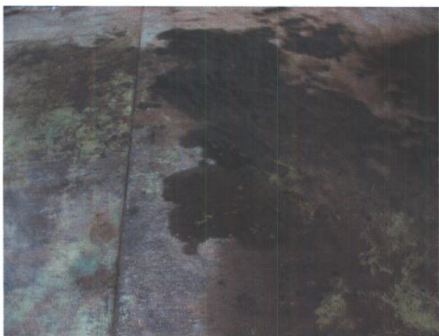
Photo #27: Oil and grease stains found in the Drill Hall.
