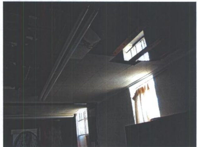
Photo #18: More missing ceiling panels located in the South Administration section.
