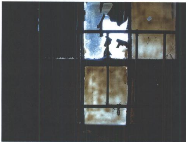
Photo #1: Peeling paint on one of the windows of the building.
