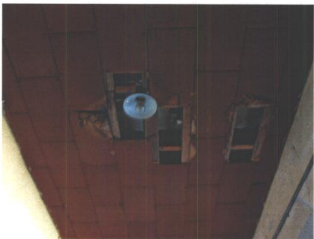
Photo #3: Missing ceiling panels in one of the rooms.
