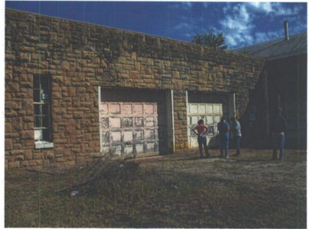
Photo #14: Motor Pool located in the west wing of the armory. Center of painting activity and area of disturbed soils.
