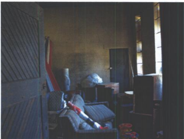
Photo #11: Room in the North Administration section of the armory controlled by Alcoholics Anonymous.
