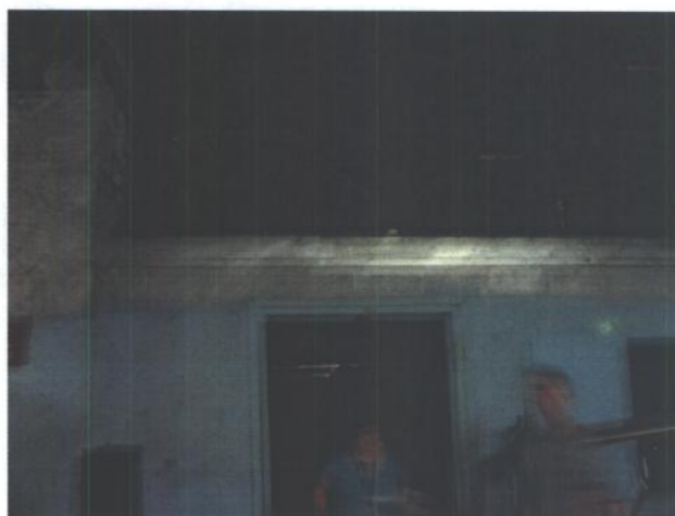
Photo #22: Possible ACM on some of the piping above a room in the in the northeast part of the South Administration section.
