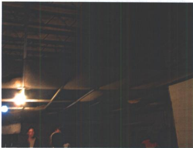
Photo #7: Missing ceiling panels in one of the rooms in the west wing of the armory.
