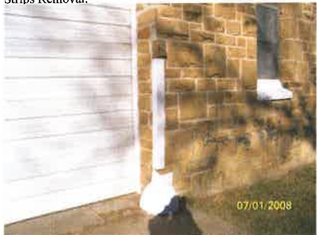
Photo: 12) Post Lead Abatement; Overhead Door Casing, Wall Trim and Window Sill after LBP.
