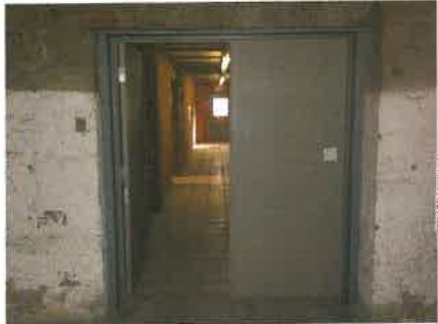
Photo: 14) Post Lead-Based Paint Abatement; New Door and Primed Door Frame after LBP Removal.
