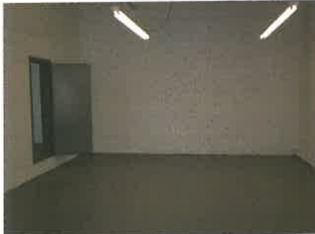
Photo: 15) Post Lead-Based Paint Abatement. Walls, Floor, Door Frame and Vault Door.
