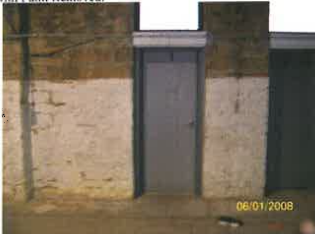
Photo: 9) Post Lead Abatement; New Door and Primed Frame after LBP removal.
