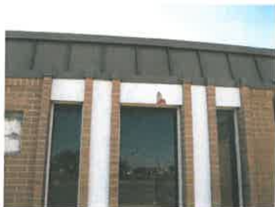
Photo # 6: White painted trim board above window - LBP.
