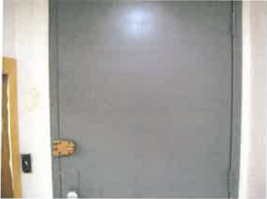
Photo #1: Gray painted door and door frame Room 14 - LBP.
