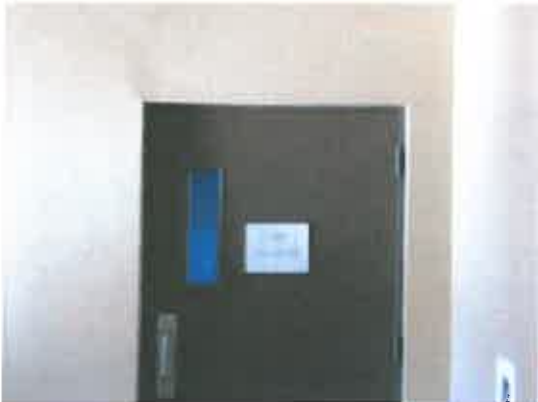
Photo #3: Brown door frame Room 5 (1) - LBP.
