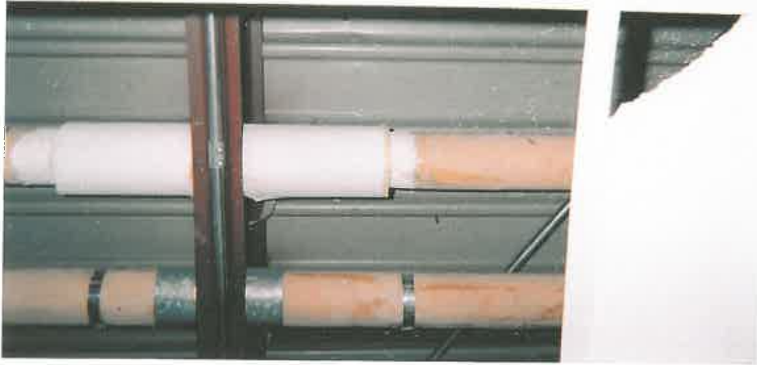
New fitting insulation
