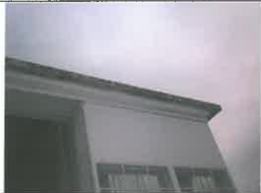
Exterior hanger door and track with LBP paint encapsulated.
