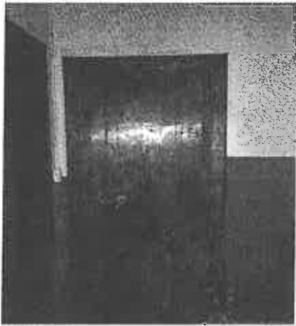
Photo: 7) Post Lead Abatement; Lead-Based Paint Door and Door Frame with Paint Removed.
