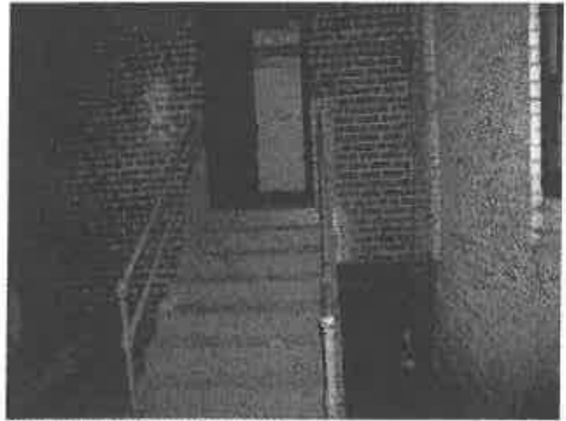
Photo: 2) Pre Lead Abatement
