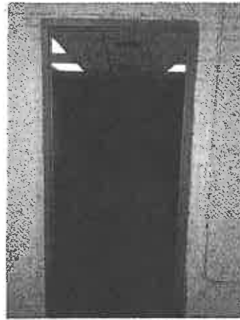
Photo: 18) Post Lead Abatement and Cleaning Activity; Primed Door Frame after LBP Removal and Floor After
