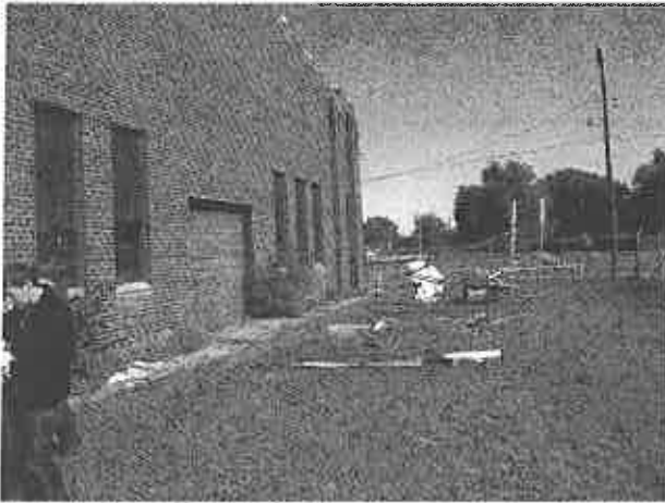
Photo: 1) Pre Lead Abatement
