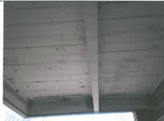
Entrance soffit ceiling deteriorated LBP to be wet scrape and encapsulate.
