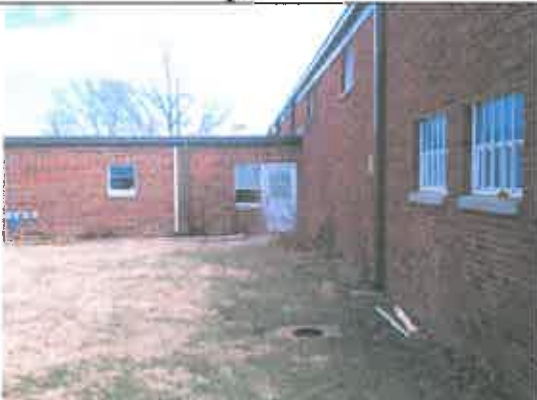
LBP door and windows to be replaced.
