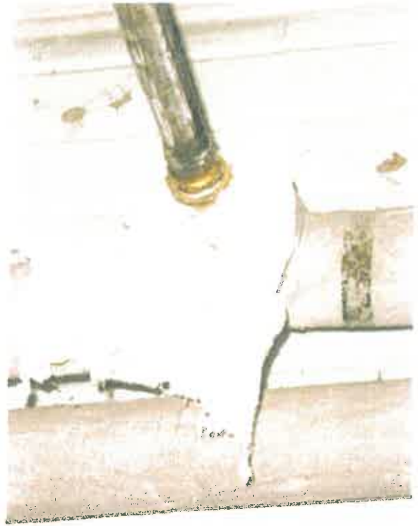
Significantly Damaged TSI in Room 10
