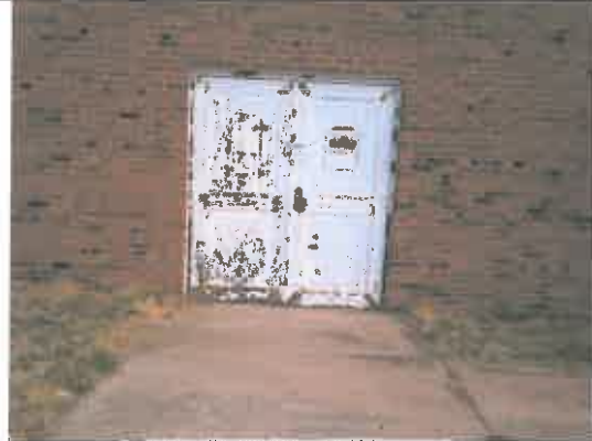
Lead-based paint door and frame to be replaced.
