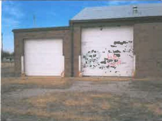
Overhead door, door frames and guard posts to be wet scrape and paint.
