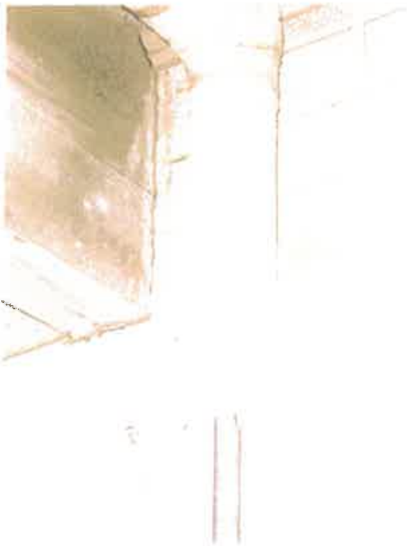
Significantly Damaged TSI in Room 10
