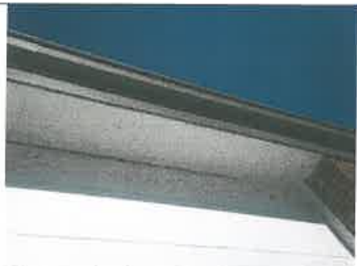
Wet scraped and encapsulated OH door frame.
