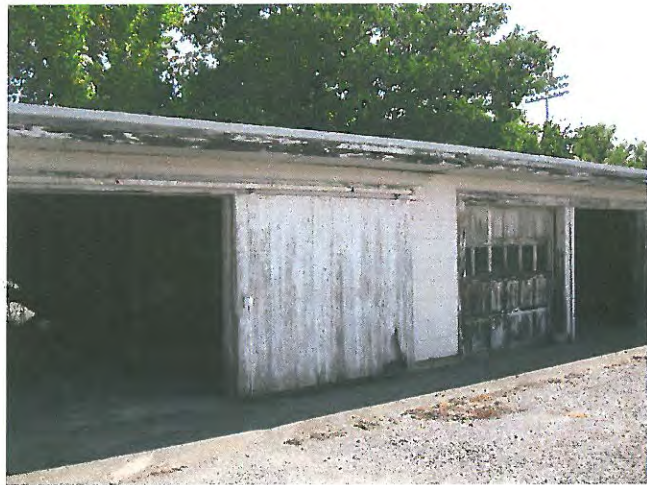
Building 4 (Lead-Based Paint and Asbestos Transite Paneling)
