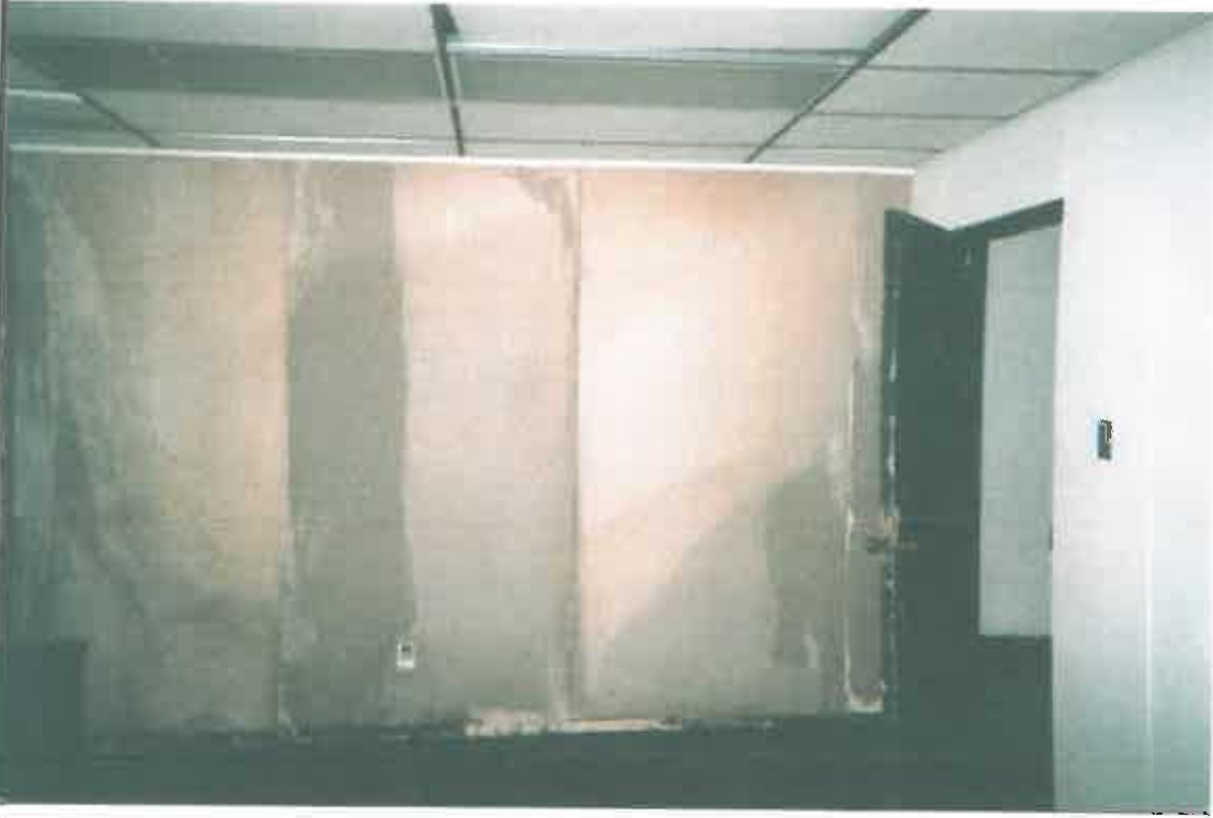
Bldg 7 - Loose and peeling paint.
