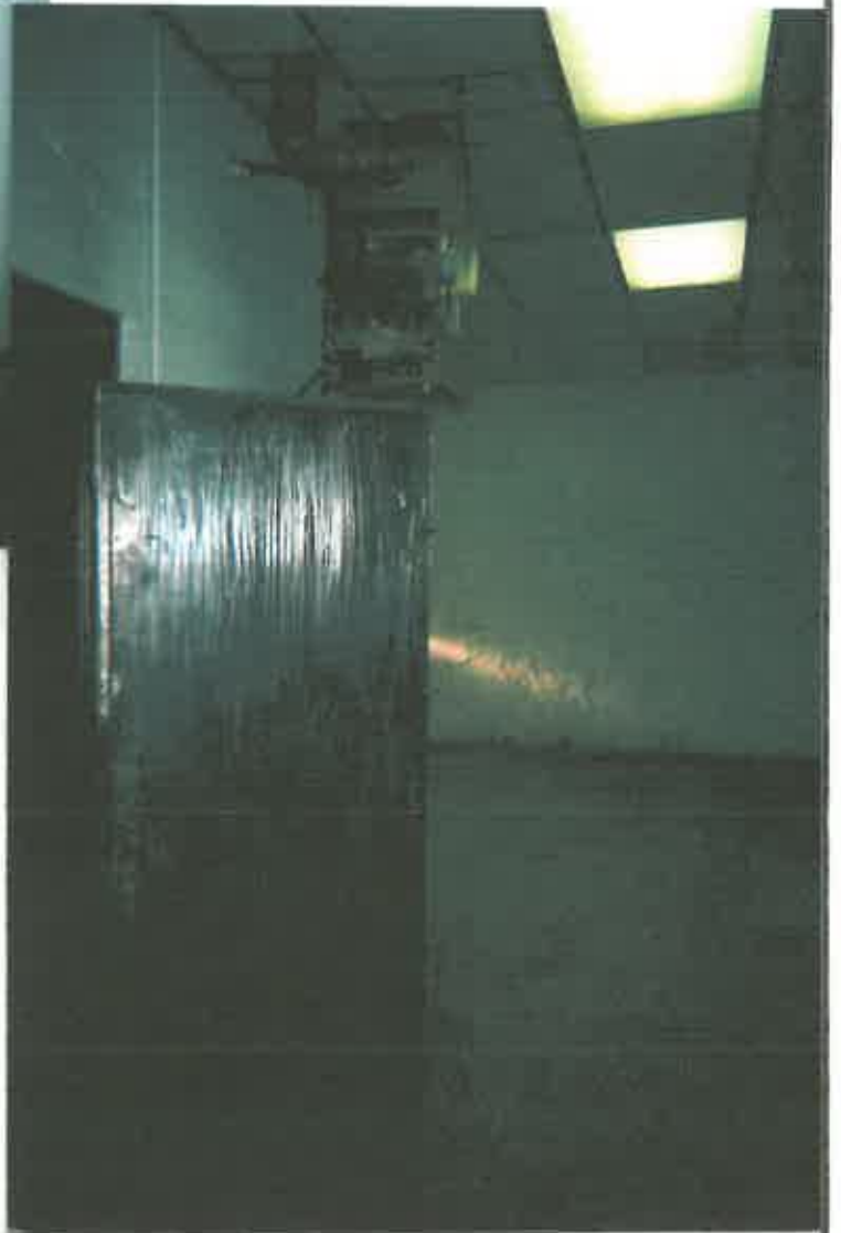
Inside of vault door after abatement of loose and peeling paint and before encapsulation.
