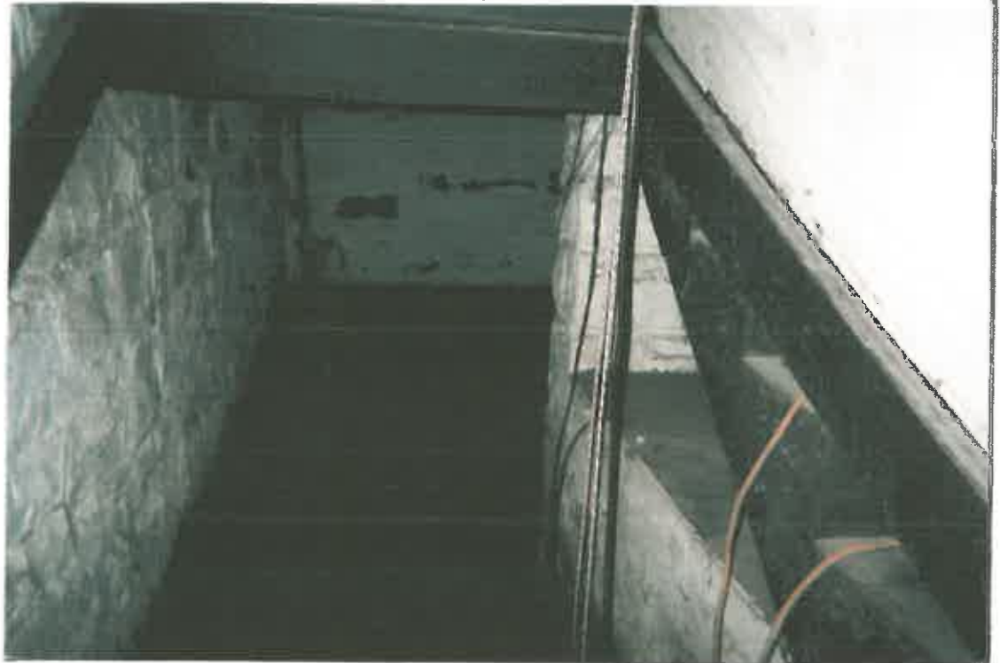
Stairwell to IFR (Water on floor).
