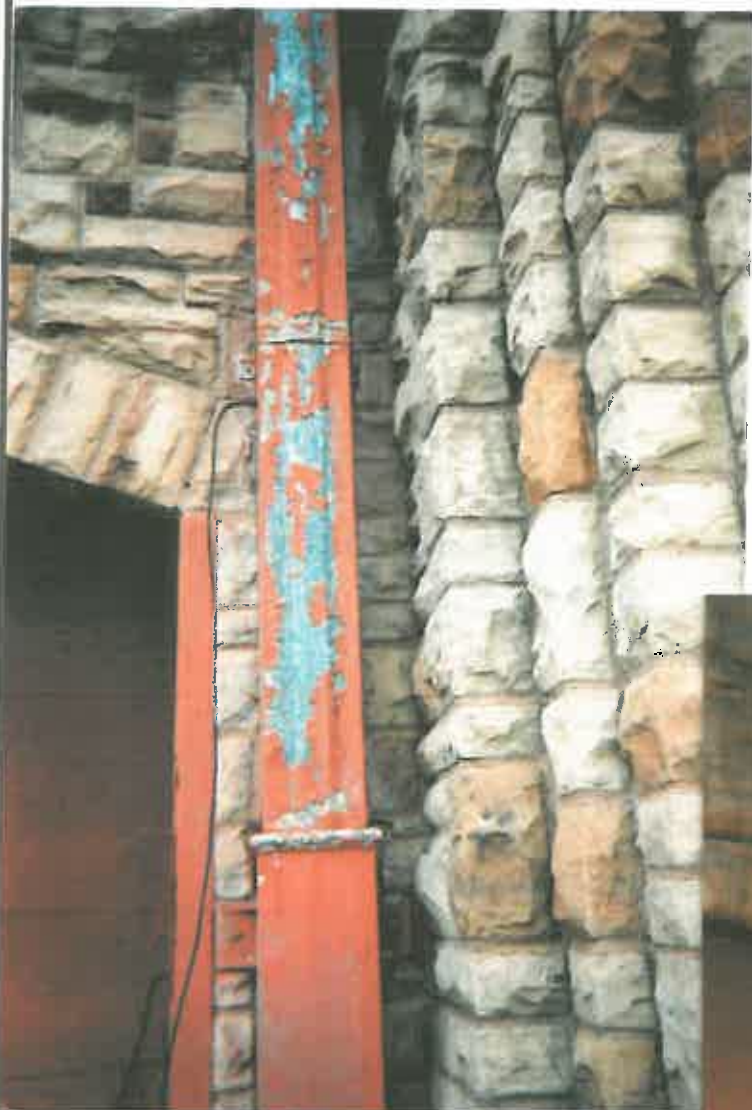
Bldg 1 - Downspout and door frame before abatement of loose and peeling paint.
