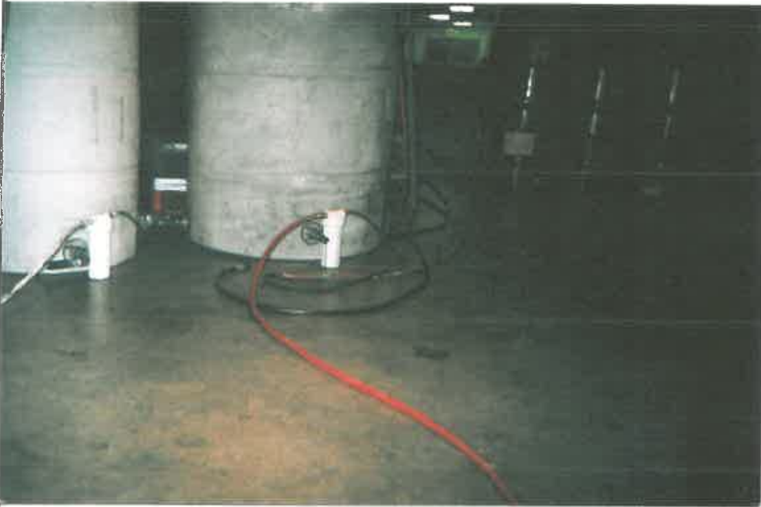
Bldg 1 - Pumps, hoses and containers for IFR water removal.
