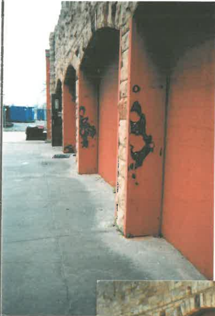
Bldg 1 - Door frame/guards before abatement of loose and peeling paint.
