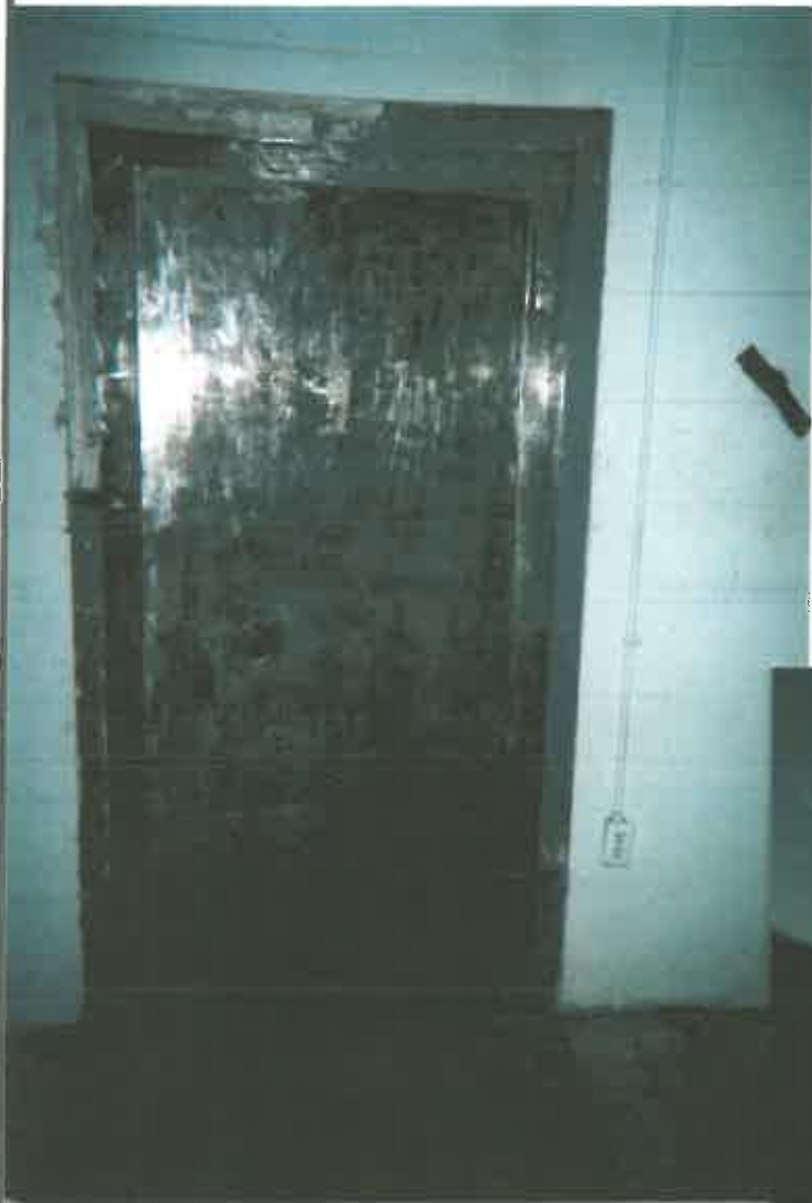
Outside of vault door after abatement of loose and peeling paint and before encapsulation.
