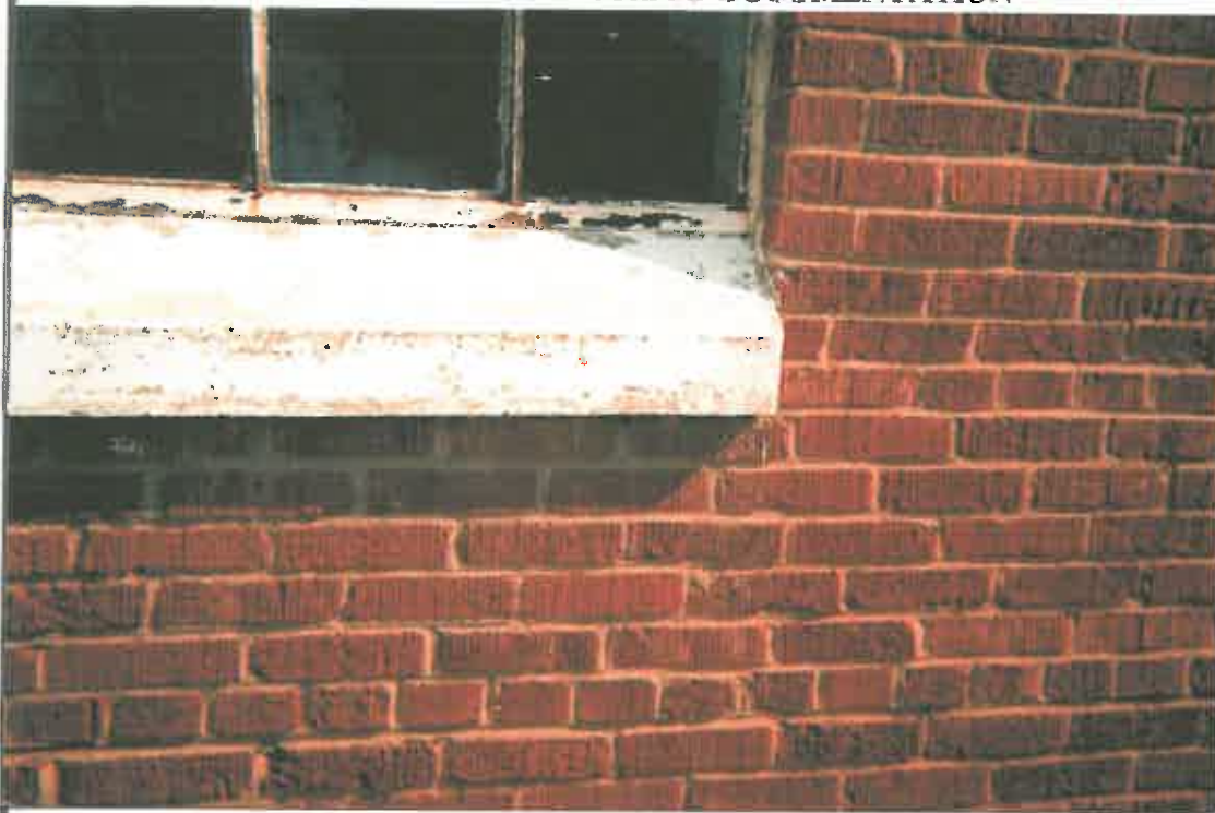
Window sill before abatement of loose and peeling paint.
