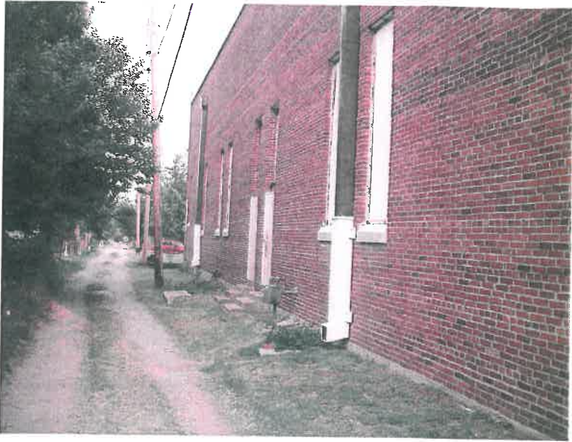
View Facing West of Alley on the South side of the Armory pre-window installation
