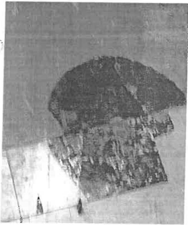
Mastic On Floor Under Tile In Rm #7 & #8
