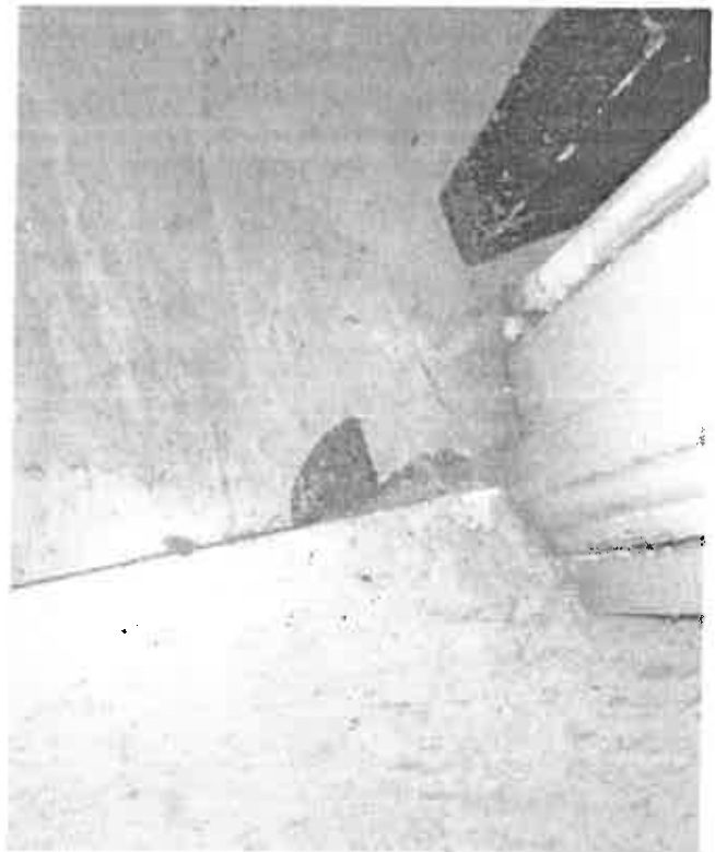
Mastic On Floor Under Tile In Room #7
