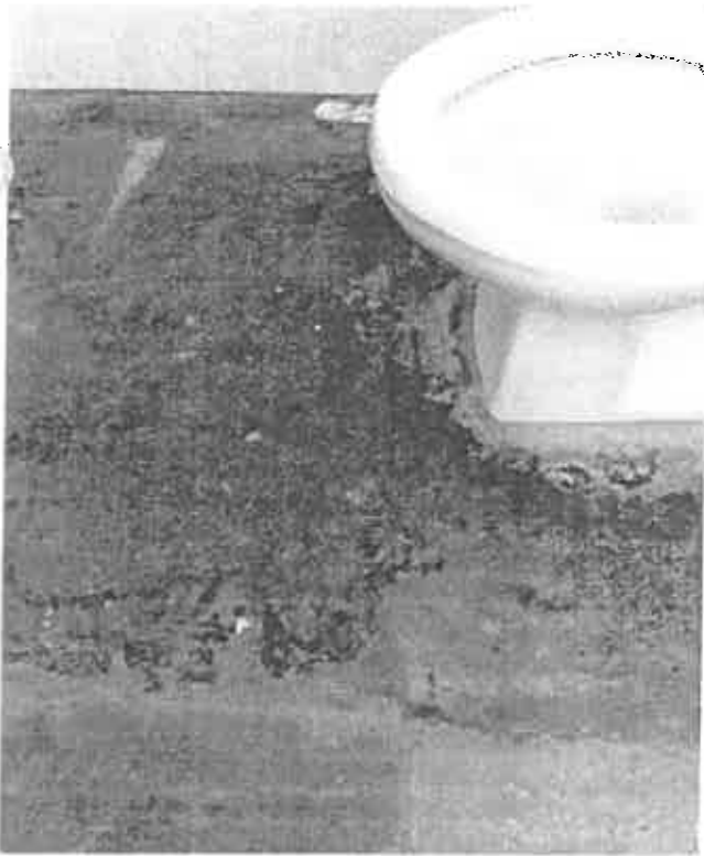
Mastic On Floor In Room #2
