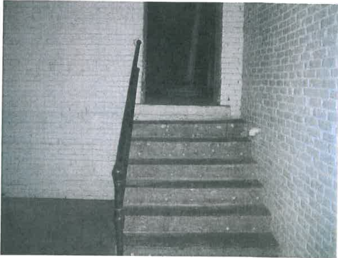
Stairs leading to entry of room # 16 prior to applying epoxy primer and encapsulant.
