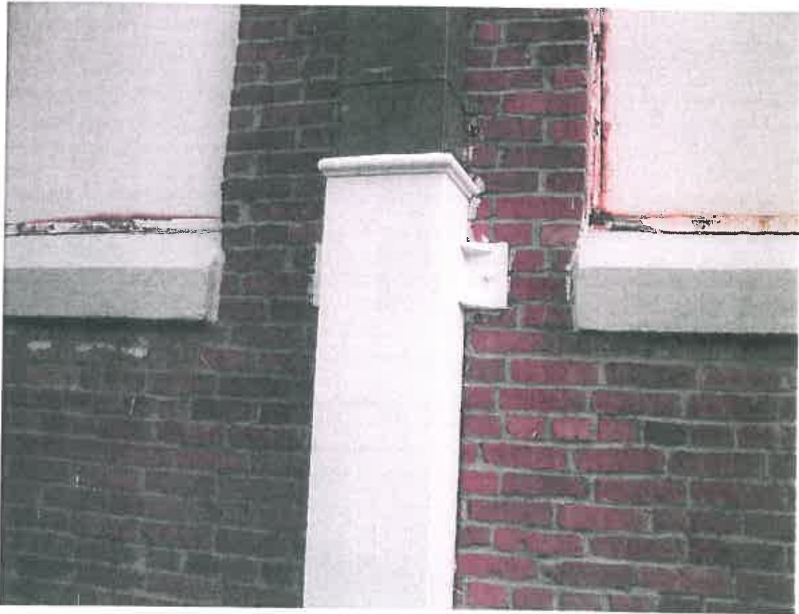
Down spout showing post wet scrape and encapsulation.
