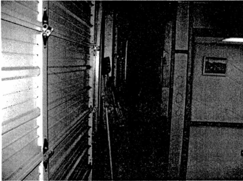
Photo 36. View of bay space behind the bay doors in the vehicle maintenance bay looking north. Note the back side of the in dining/classroom area walls adjacent to kitchen.
