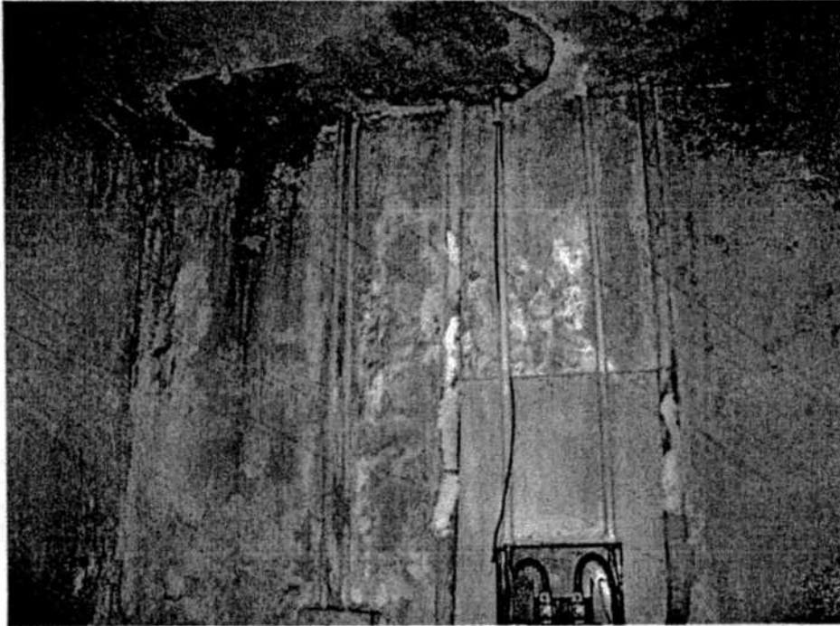
Photo 48. Water damage on southeast wall of room located off the southeast corner of the drill floor.
