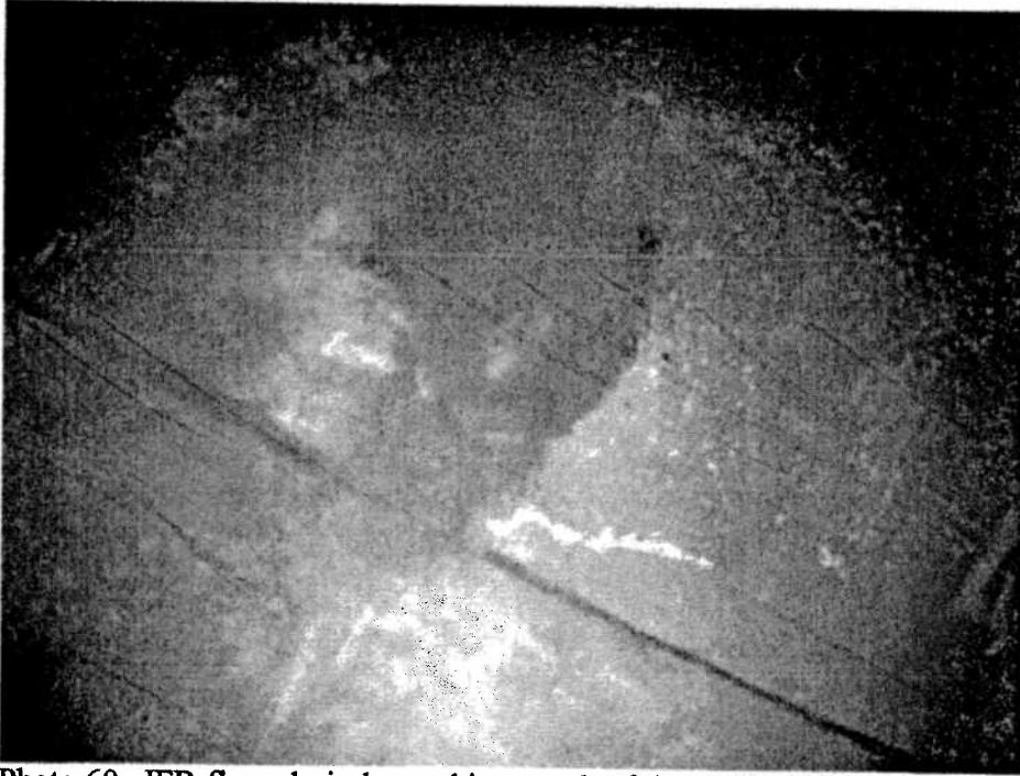
Photo 60. IFR floor drain located just south of the center of the IFR.
