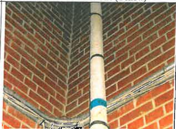
HA #8: Pipe Insulation (Cold)
