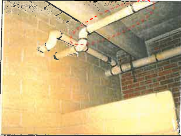
HA #9: Piping Insulation (Hot)
