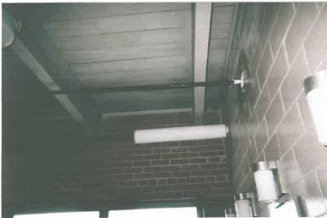
HA #8 & #9: PIPE INSULATION ABATED, PIPE "LOCKED DOWN" AND WALL PENETRATIONS SEALED. NON-ACM INSULATION REPLACEMENT INITIATED.
