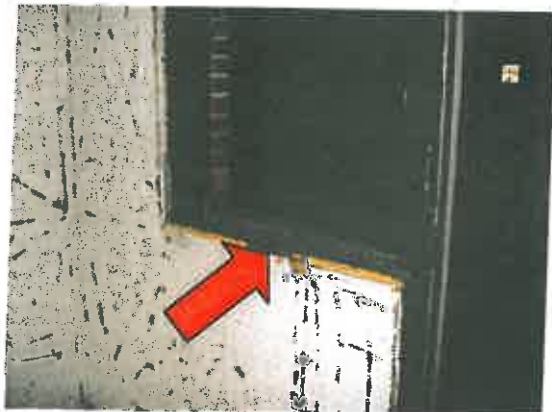
Photo # 5: Black painted pass through window sill in Room 14 - LBP.
