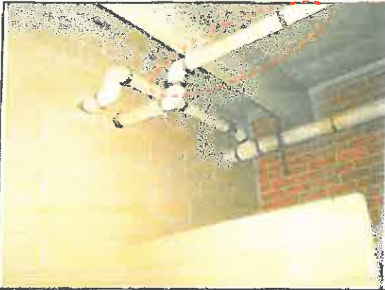
HA #9: Piping Insulation (Hot)
