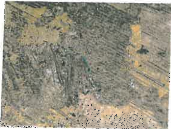
Photo #3: View of green painted concrete floor in Room 6 - LBP.
