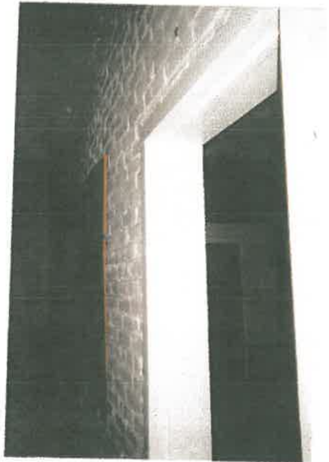
ABATED AND SEALED DOOR FRAME
