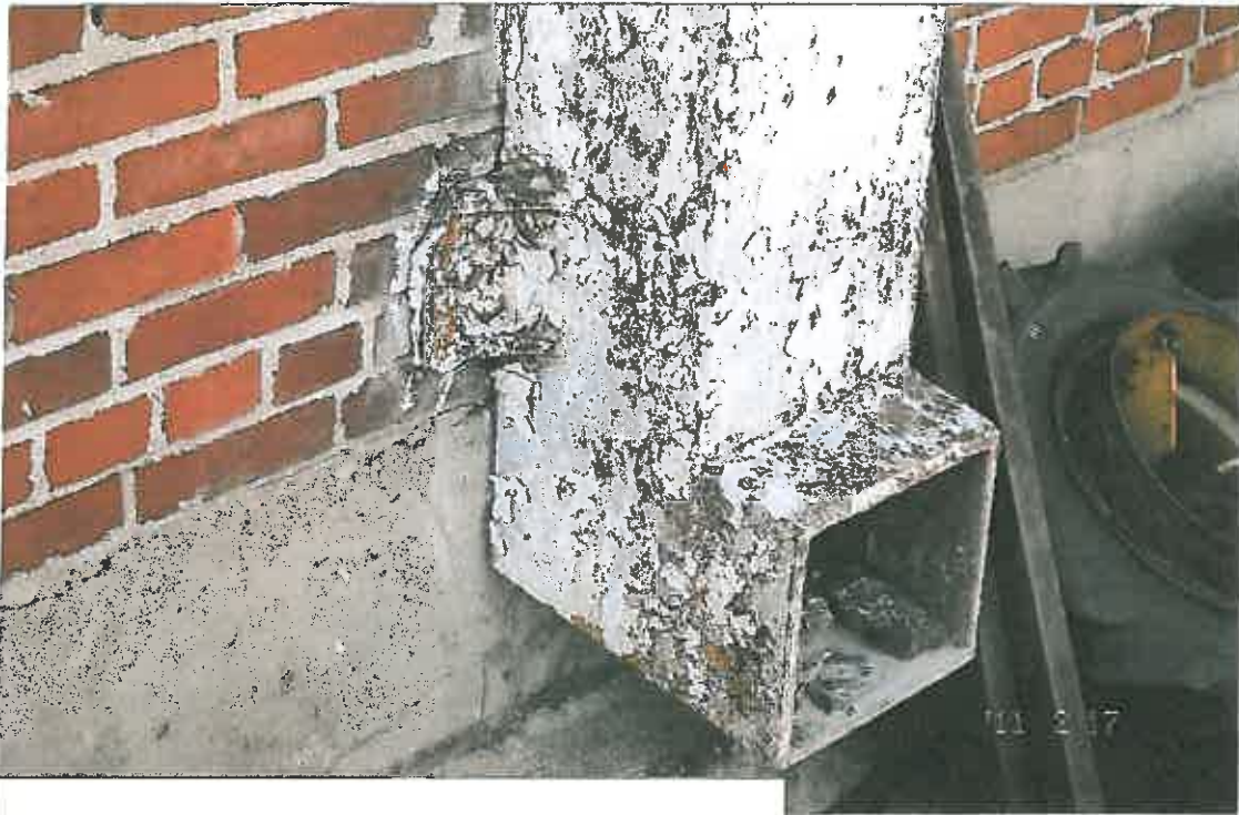
LOOSE AND PEELING PAINT ON DOWNSPOUT
