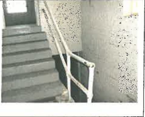
Room 8 - Side C - Stair Rail
