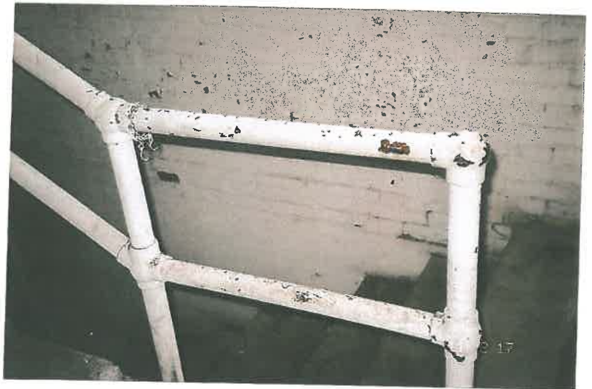
LEAD BASED PAINT ON HANDRAIL
