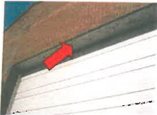
Photo #3: Lintel above roll-up door - LBP.
