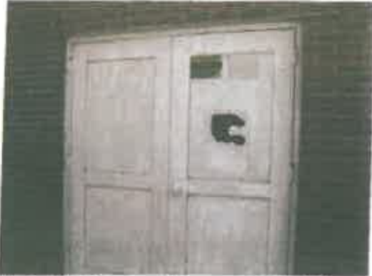
Photo #7: Door and frame and intel Side C Exterior - LBP
