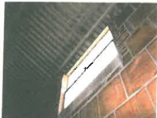
Photo #10: High bay window in Room 1 - LBP
