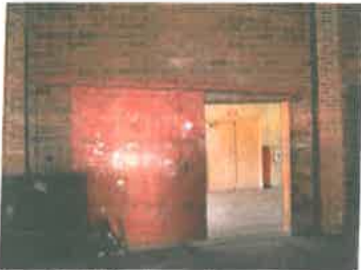
Photo #9: Sliding door and track on Side C of Room 1 - LBP.
