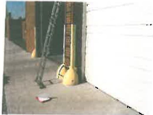
Photo #2: Modified bollards and edge protectors - LBP.
