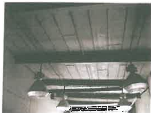
Photo #12: Kaylo ceiling in Room 2 - LBP
