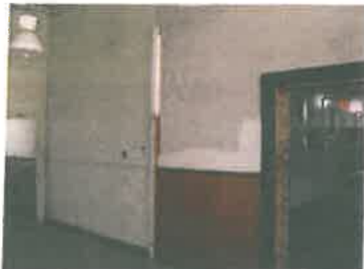
Photo #11: Walls, door frame, wall trim, and baseboard-Room 2 - LBP.
