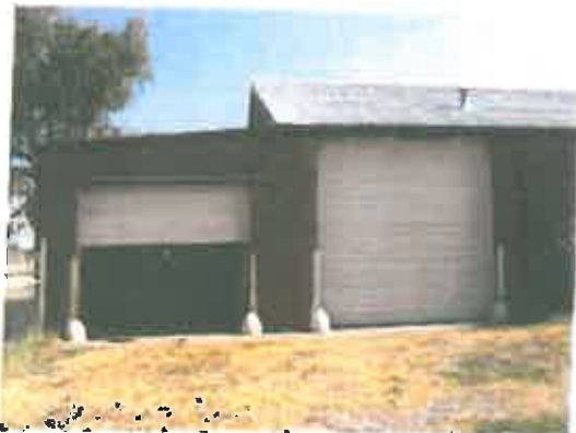
Photo # 5: Modified bollards and edge protectors - LBP.
