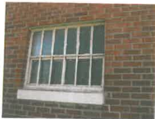
Photo # 6: Window frame and lintel - LBP.
