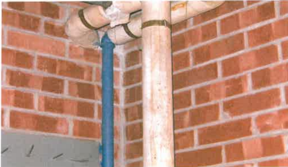
Friable Asbestos Containing Pipe Insulation
