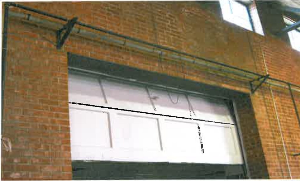
Friable Asbestos Containing Pipe Insulation
