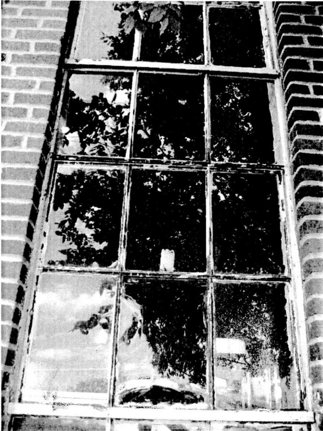
Figure 4: Healdton Armory – south window on outside west wall with chipped paint.
