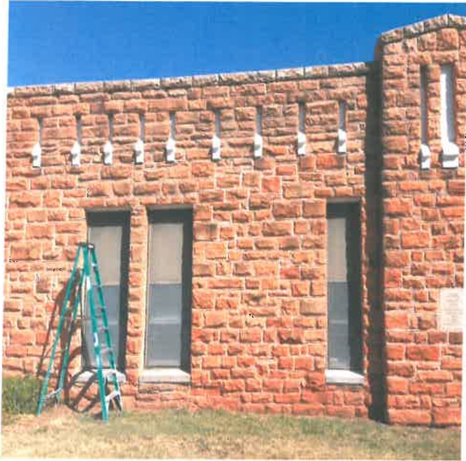
Typical masonry after lead base paint stabilization.
