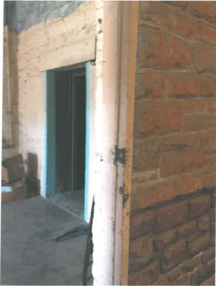
Typical original condition of a painted metal door jamb.
