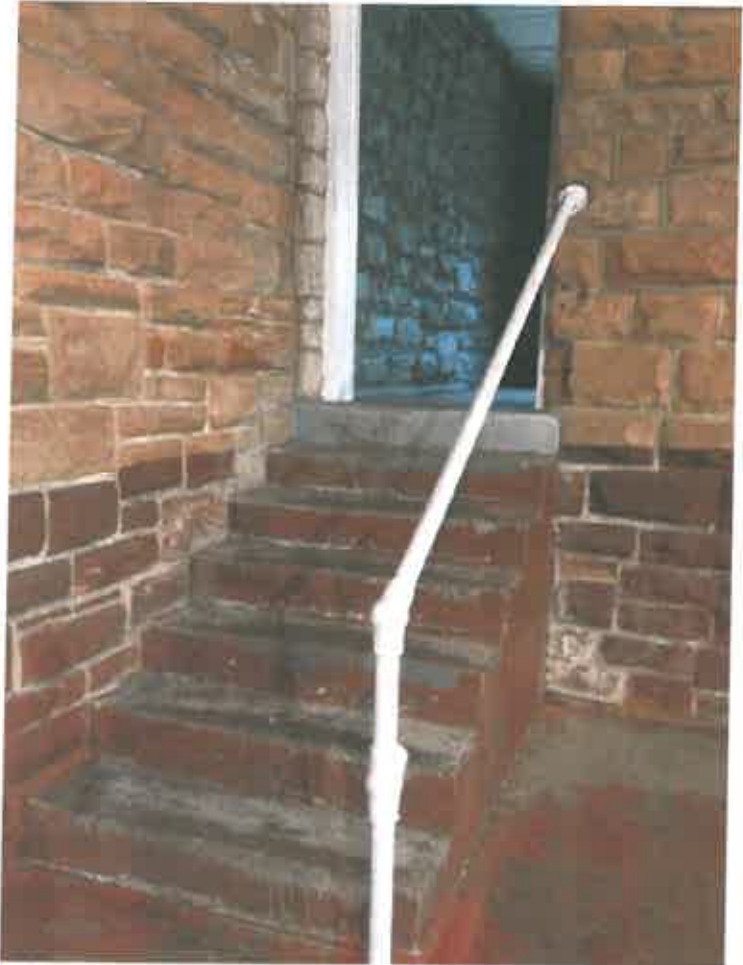
Typical conditon of a primer handrail.
