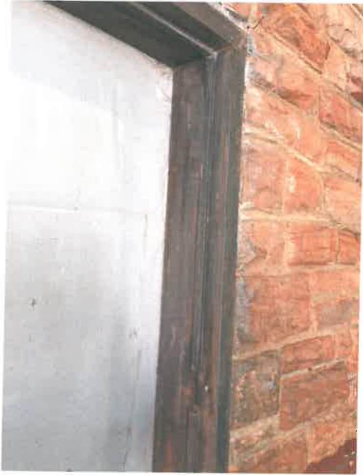
Typical condition of a striped metal door jamb
