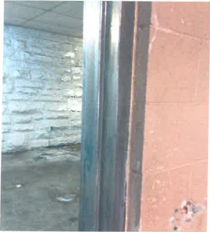
Typical conditon of a striped metal door jamb
