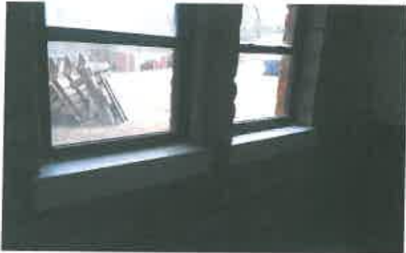
Typical interior window sills that have been cleaned and had primer applied.
