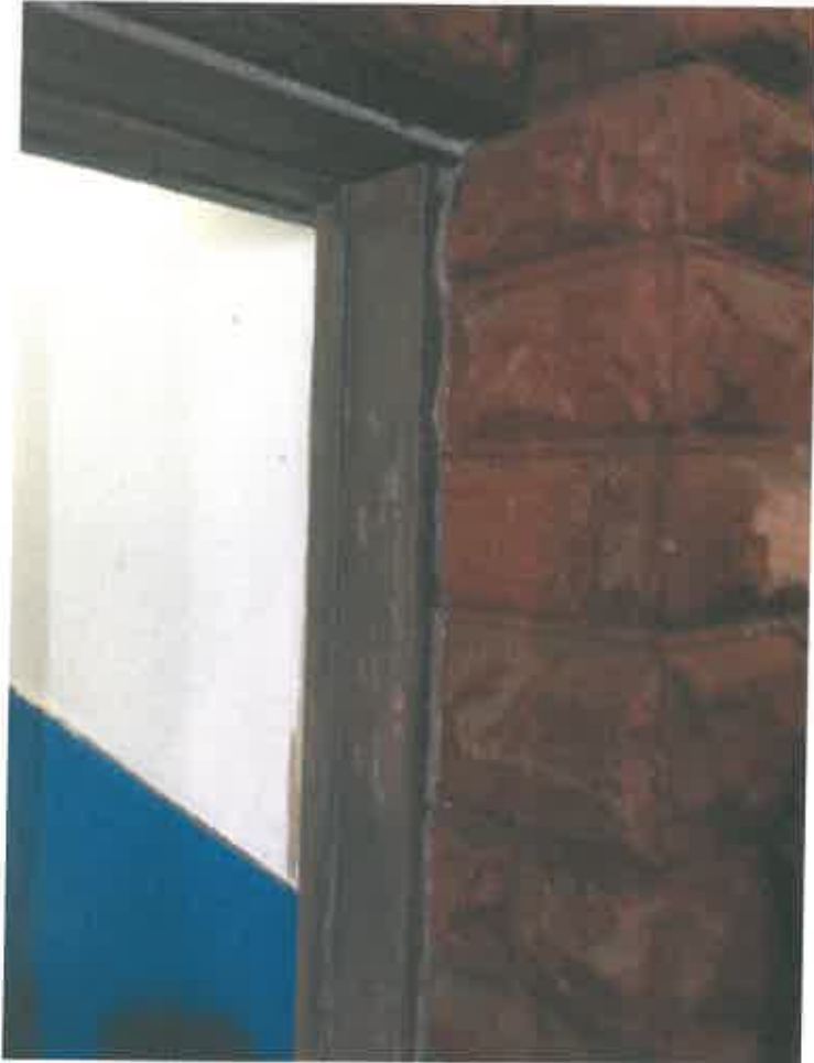
Typical conditon of a striped metal door jamb
