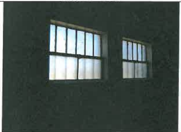
Photo #5: Gray/Brown Window Frame Room 2 – LBP.
