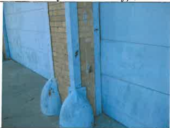
Photo #8: Gray Edge Protector and Modified Bollard Side A Exterior – LBP.
