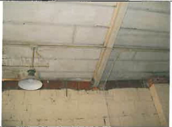
Photo #4: Gray Ceiling Deck Room 2 – LBP.
