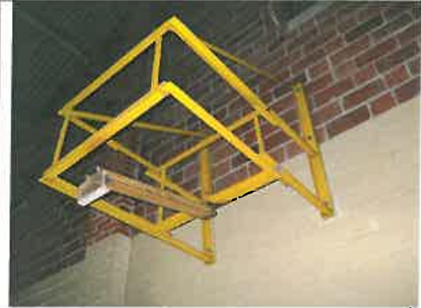
Photo #3: Yellow Basketball Goal Frame Room 1 – LBP.
