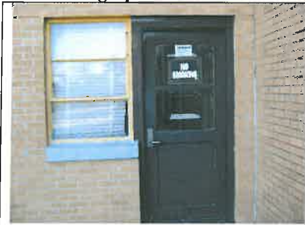
Photo #7: Yellow Window Frame and Brown Door and Frame Side C Exterior-Room 3 – LBP
