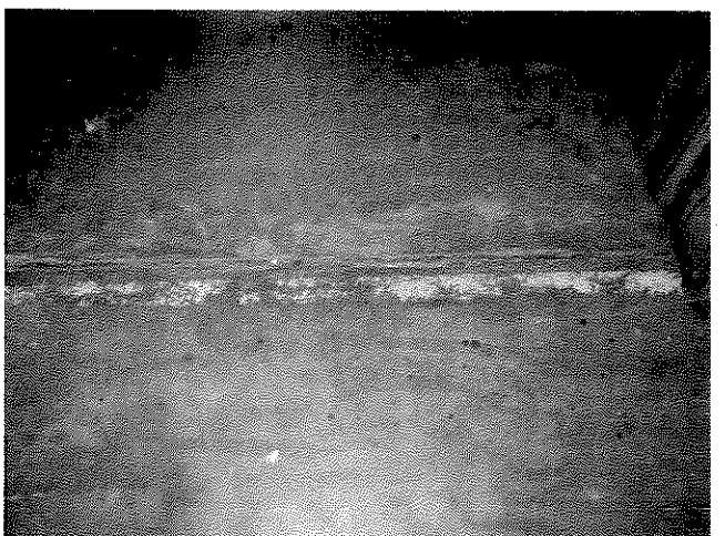
Photo #24: Yellow primer located on the surface of the Drill Floor
