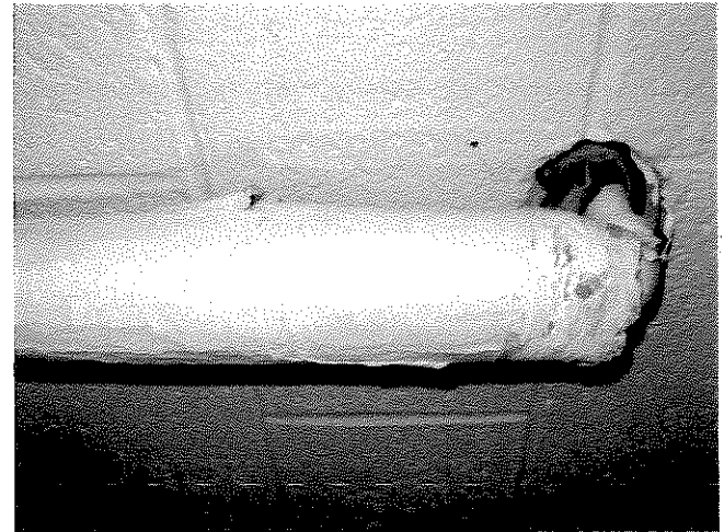
Photo #18: Close-up view of the TSI, which may contain ACM
