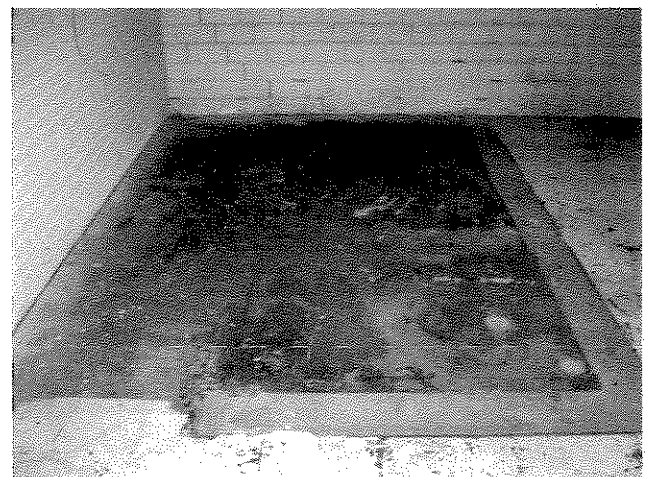
Photo #12: Red primer located on the floor of the Maintenance Area
