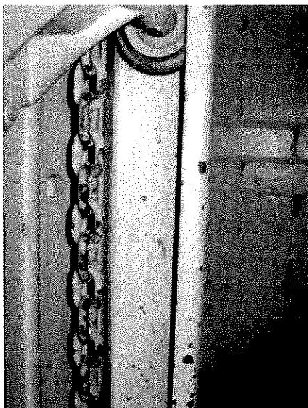
Photo #11: Suspect lead-based paint on an overhead door
