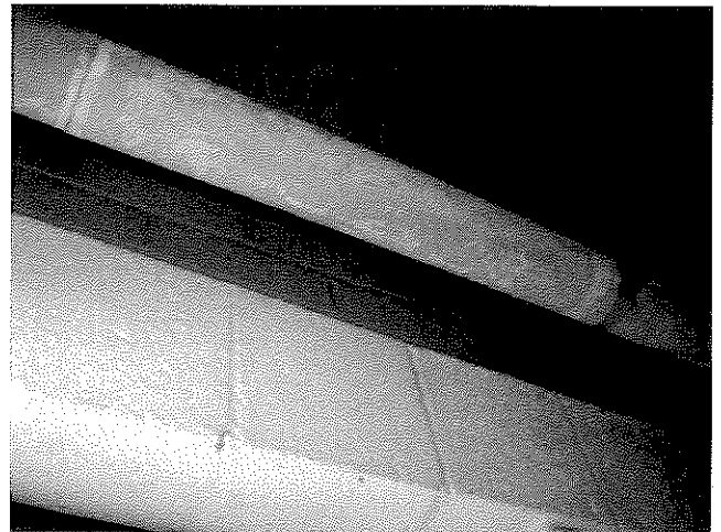
Photo #20: Green-colored metal surface pipe inside the Supply Room
