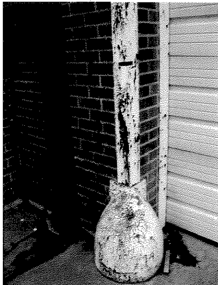
Photo #5: Corner metal siding near an overhead door
