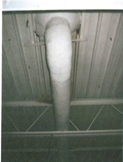
Photo #41: TSI in Section Room
