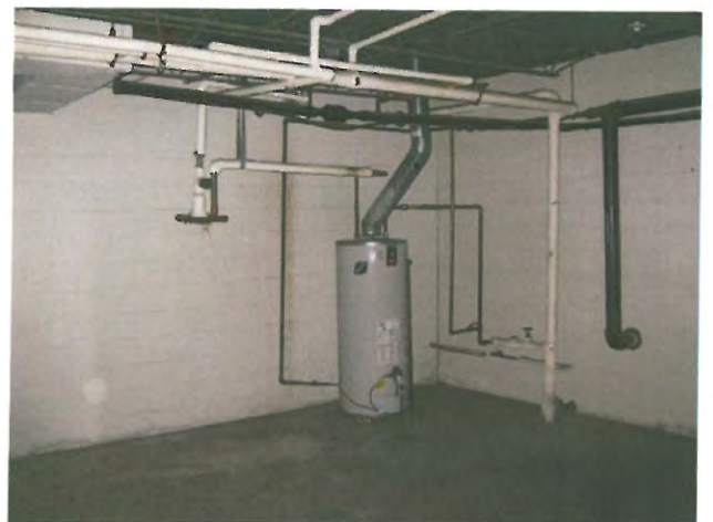
Photo #24: Boiler Room with TSI
