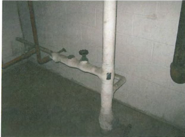
Photo #25: TSI inside the Boiler Room
