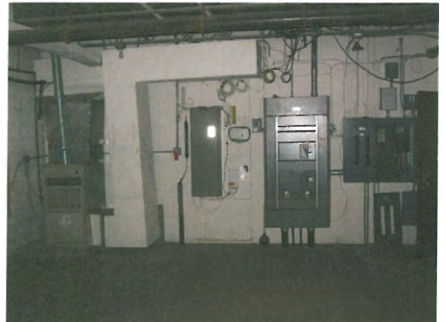
Photo #26: Circuit Boards and furnace inside the Boiler Room.
