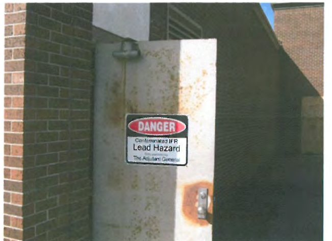
Photo #6: IFR door with lead hazard sign
