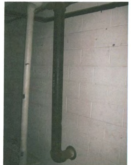
Photo #29: TSI in Boiler Room
