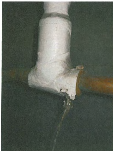
Photo #28: TSI in Boiler Room
