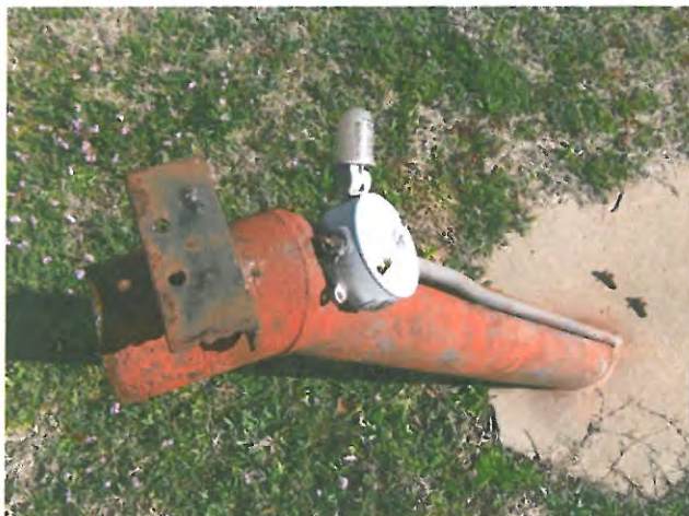
Photo #11: Utility meter located northwest of the Armory.
