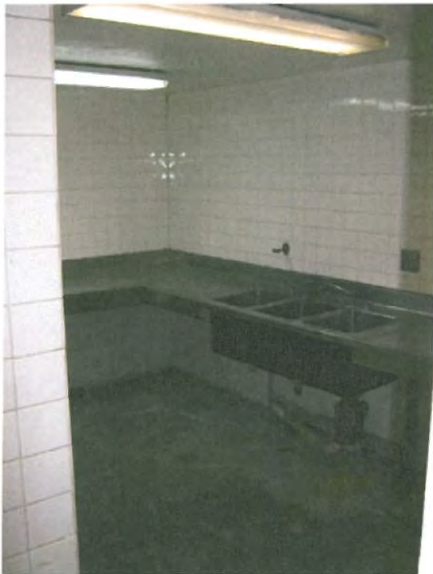
Photo #44: Sink in Kitchen with exposed mastic
