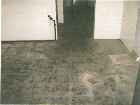
Photo #46: Exposed mastic in Kitchen
