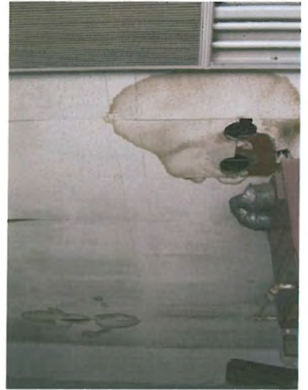
Photo #61: Water Damage inside IFR ceiling.
