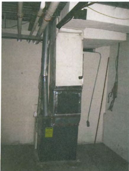
Photo #27: TSI in Boiler Room
