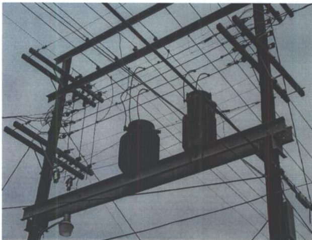
Photo #15: Close-up view of the pole-mounted transformers.
