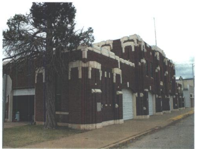
Photo #8: View of the north and northeast corner of the armory building.
