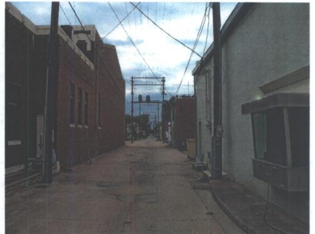
Photo #16: Pole-mounted transformers located southwest of the armory building.
