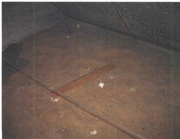
Photo #23: Close-up view of the IFR sand trap.
