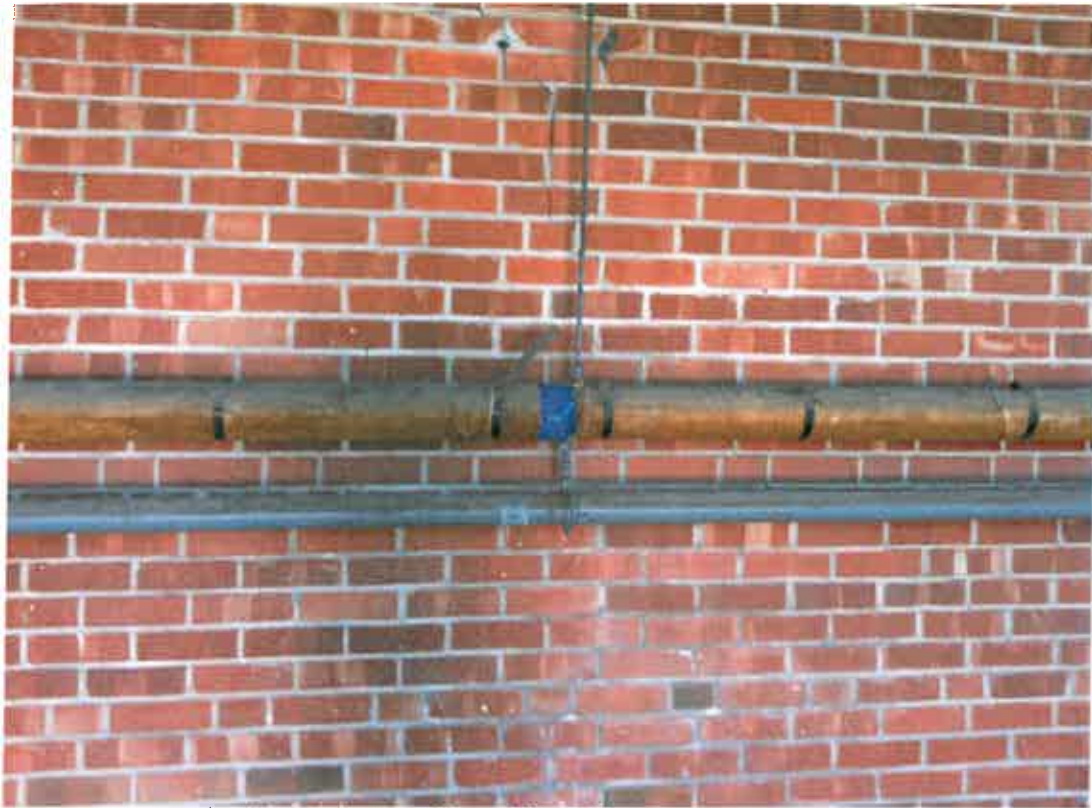
Friable Asbestos Containing Thermal Pipe Insulation (Sample # BA-17C)
