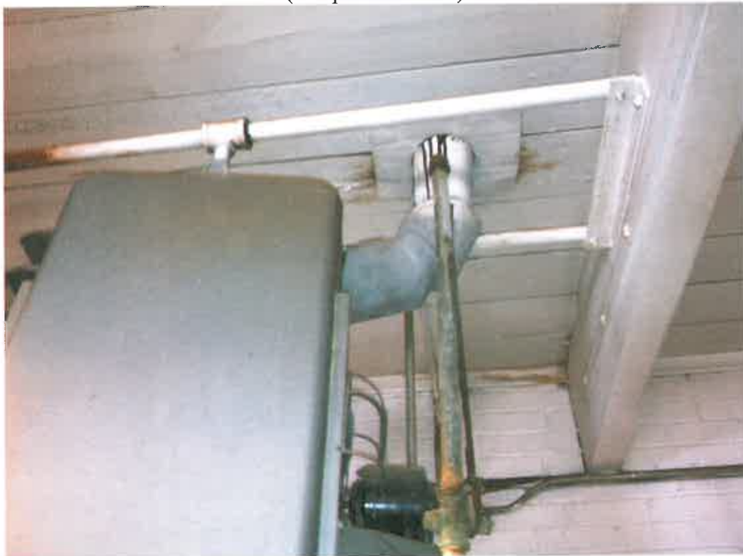
Non-Friable Transite Heater Vent Pipe (Not Sampled)
