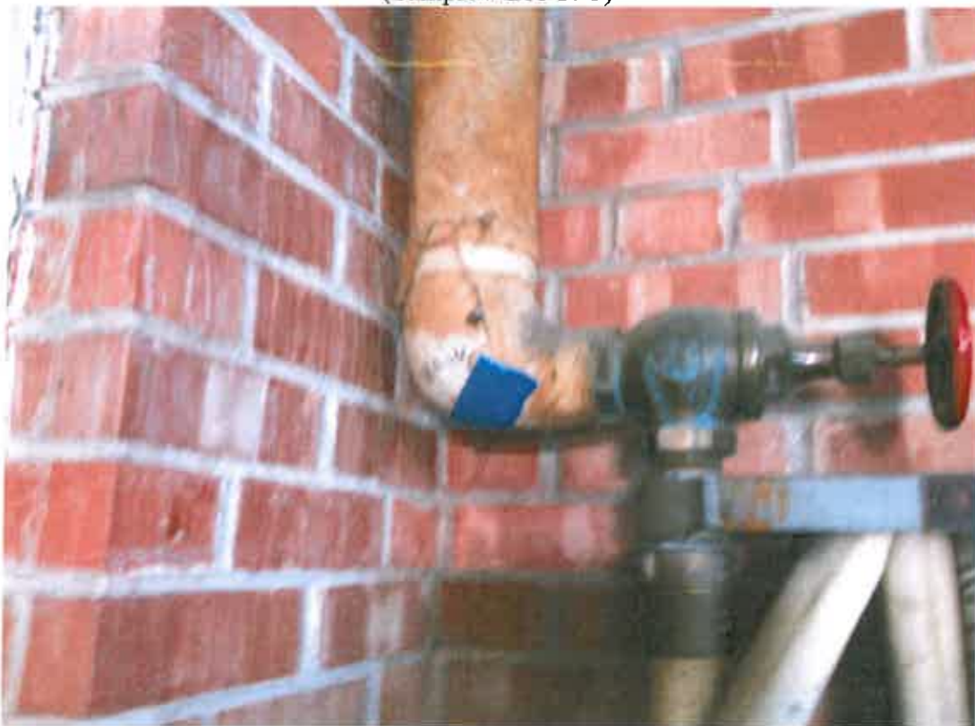
Friable Asbestos Containing Thermal Pipe Fitting (Sample # BA-18C)
