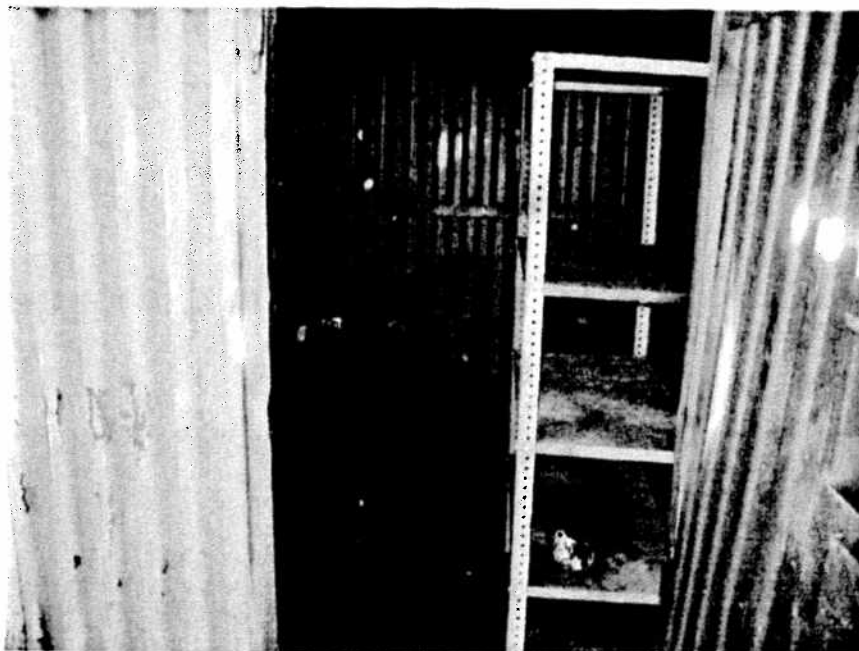
Figure 19. Flammable liquid storage box in the southwest side of vehicle impoundment near IFR bay door.
