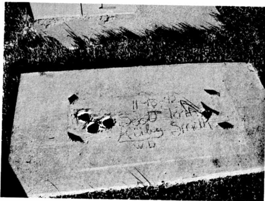
Figure 13 Concrete pad south of transformer box on east side of building. Note open conduit piping - facing north.
