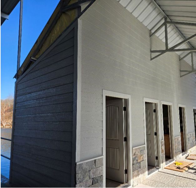
Photo Series #2 Burnt Cabin Marina December 19, 2024 Floating restrooms
